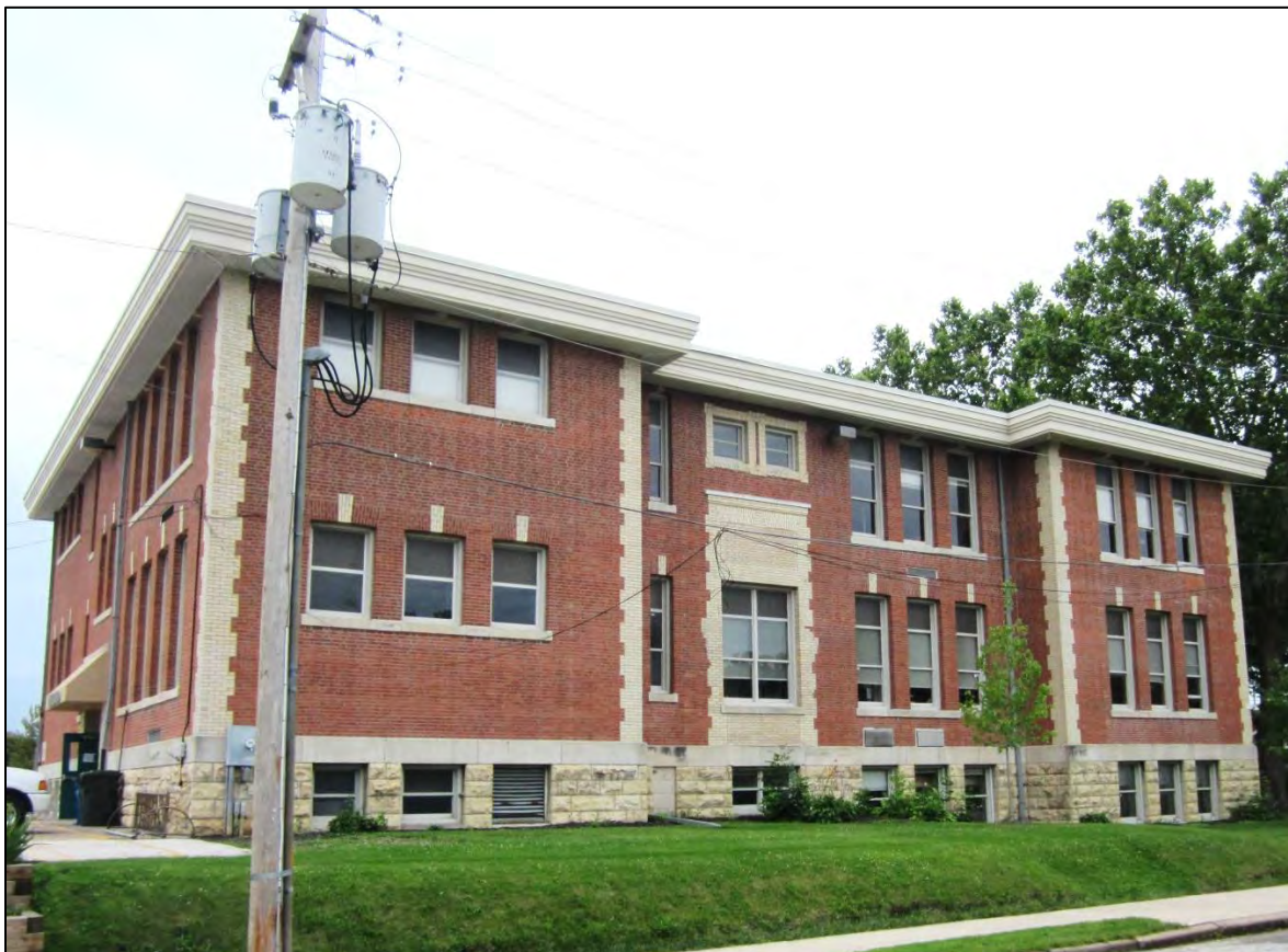
Figure 14: Current photograph (2015) of the Willard School, showing the altered roof line and non-historic cornice on the east elevation
