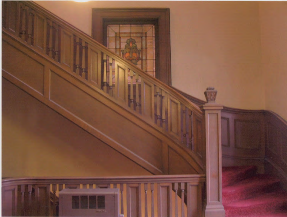
Photo #27 (WA_KingCounty_FirstUnitedMethodistChurch_0027) Front Stairwell Vestibule – Typical guardrail, handrail, wainscott & stained glass window
