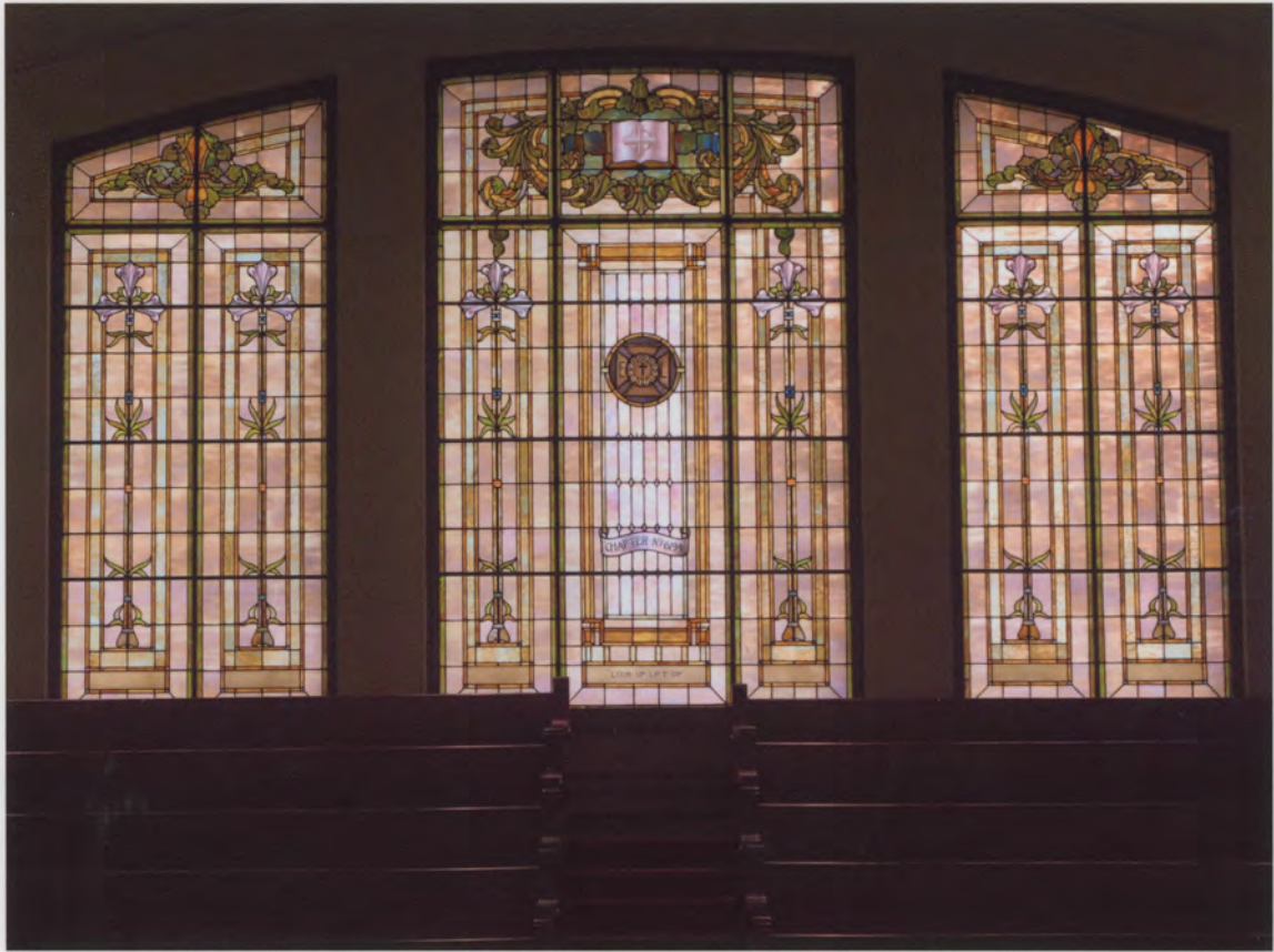
Photo #33 (WA_KingCounty_FirstUnitedMethodistChurch_0033) Stained Glass Windows (Main Auditorium) above gallery at north wall
