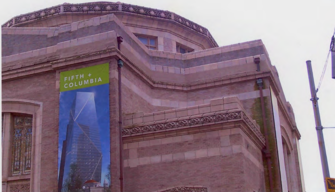
Photo #13 (WA_KingCounty_FirstUnitedMethodistChurch_0013) Exterior Detail – Typical main cornice (missing) & parapet with intact dome cornice above (K. Krafft 5-16-10)
