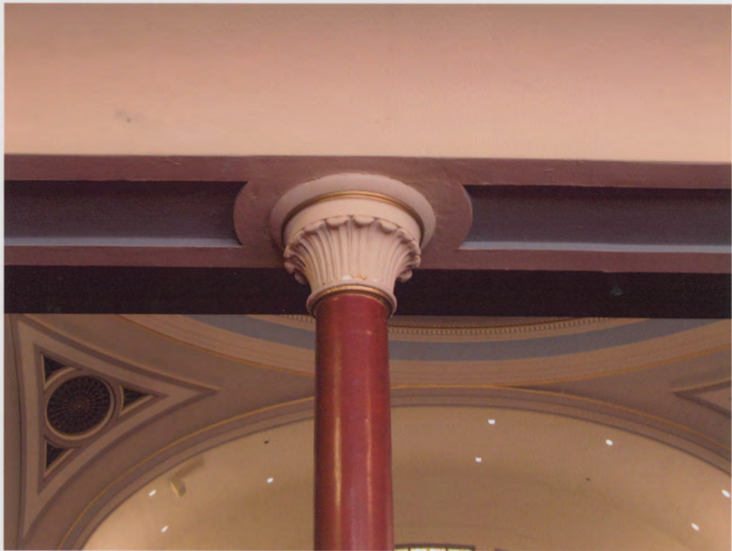
Photo #22 (WA_KingCounty_FirstUnitedMethodistChurch_0022) Main Auditorium – Detail – typical cast iron column w/ fluted capital
