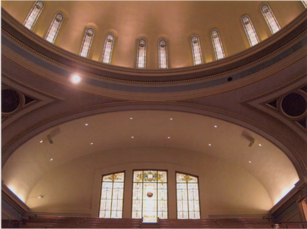
Photo #25 (WA_KingCounty_FirstUnitedMethodistChurch_0025) Auditorium Dome – view east of light cove cornice and clerestory windows
