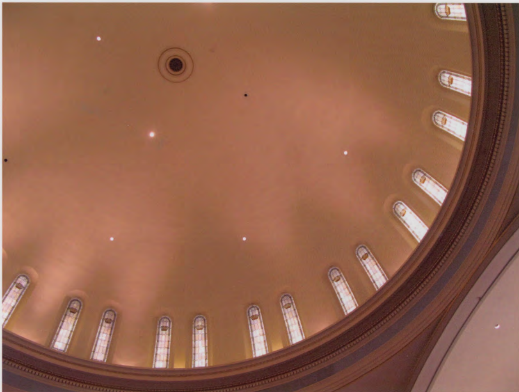
Photo #26 (WA_KingCounty_FirstUnitedMethodistChurch_0026) Auditorium Dome – view from below of light cove and clerestory windows
