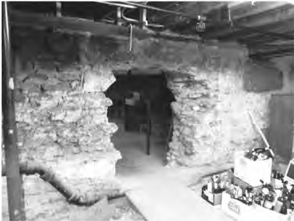
Figure 7 - Doorway cut through north foundation wall of the c. 1862 building, leading into the 1893 north bay basement.
