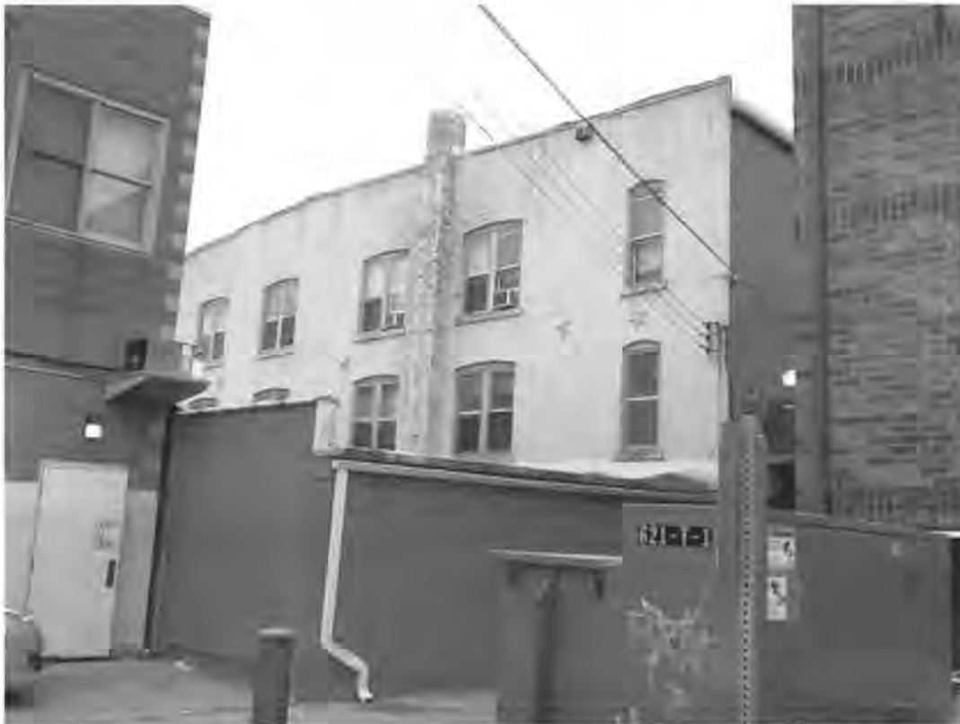
Figure 6 – North side wall. The rear alley side is on the right. The small midcentury commercial building that houses a hairdresser’s salon, painted dark red here, obscures the ground floor of this 1893 bay addition to the Union Bakery.
