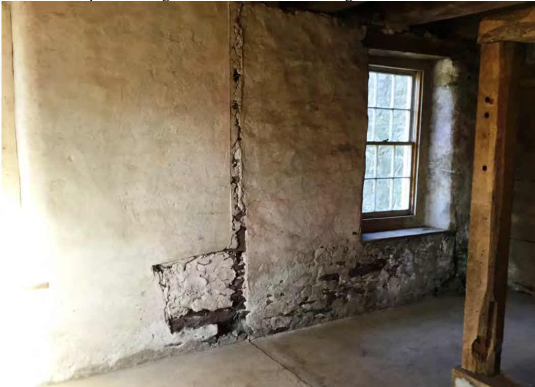
Barn interior photo 17 of 17. Stable level removed wall for cattle stalls. Trough scar visible on wall
