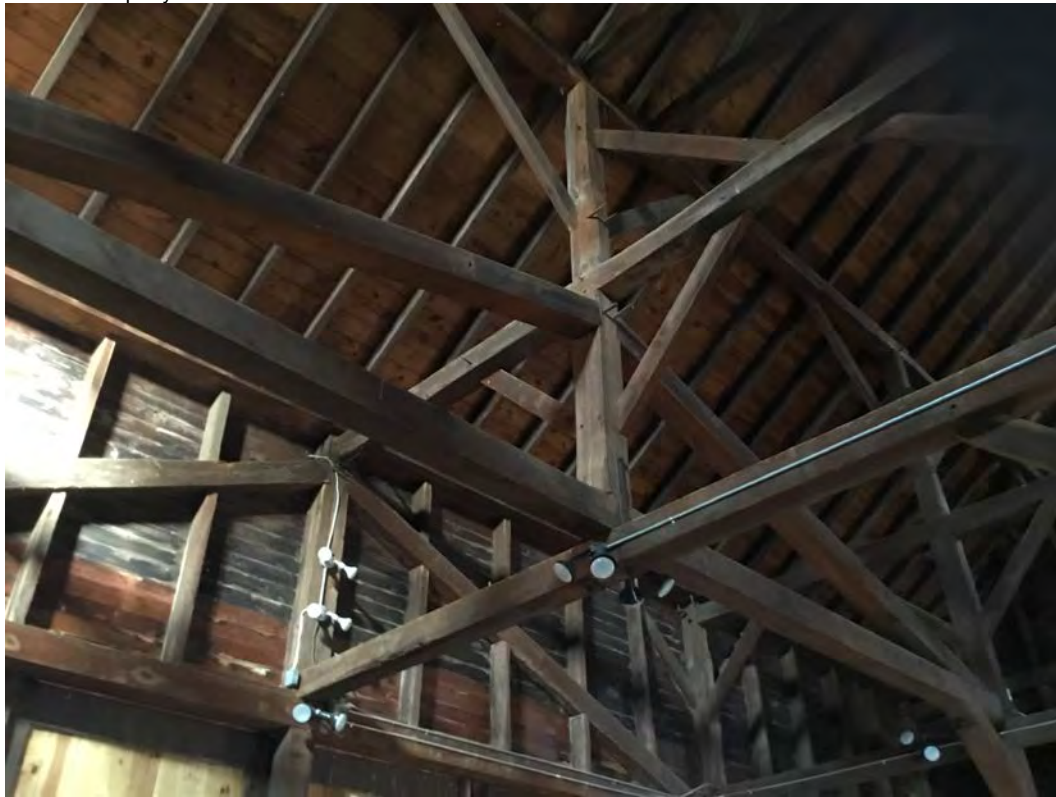
Barn interior photo 10 of 17. King post trusses above threshing bays facing northeast.
