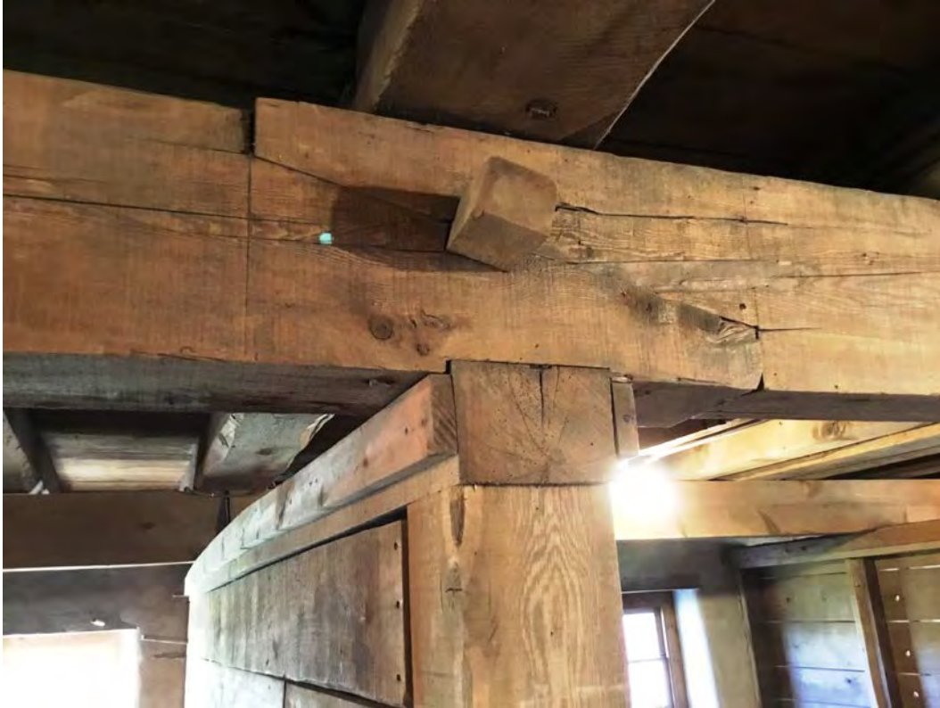
Barn interior photo 14 of 17. Stable level summer beam with keyed scarf joint facing south
