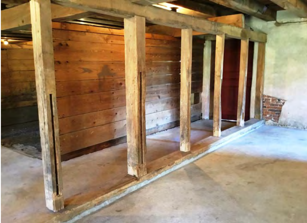
Barn interior photo 16 of 17. Stable level removed partitions for cattle stalls. Partitions inset into slots into the posts. Trough scar visible on wall facing south
