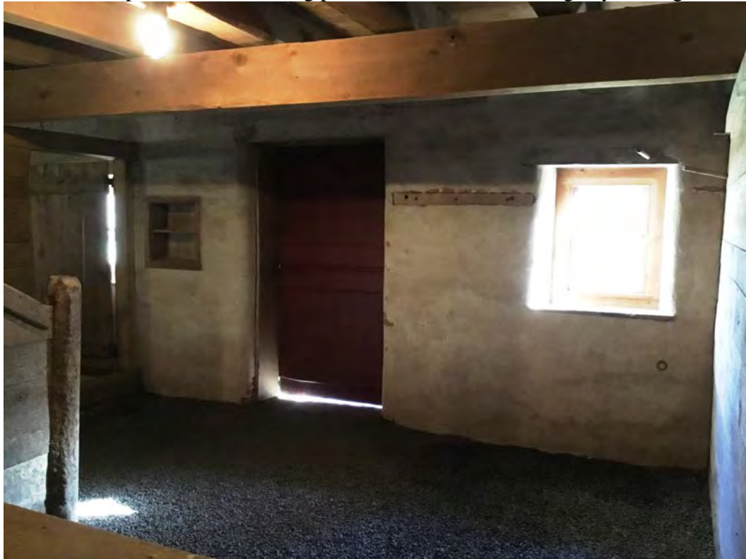
Barn interior photo 11 of 17. Stable level stall wall with curry comb niche and tack rack (pegs removed) facing south
