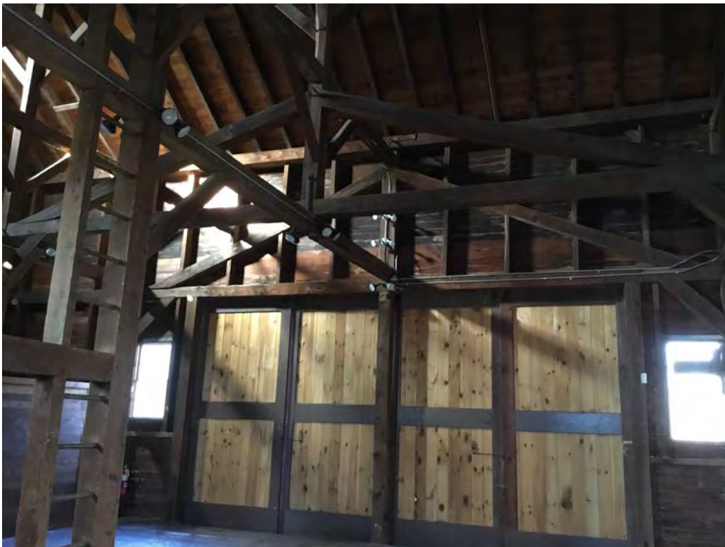
Barn interior 5 of 17. Post in east gable with wicket holes facing west
