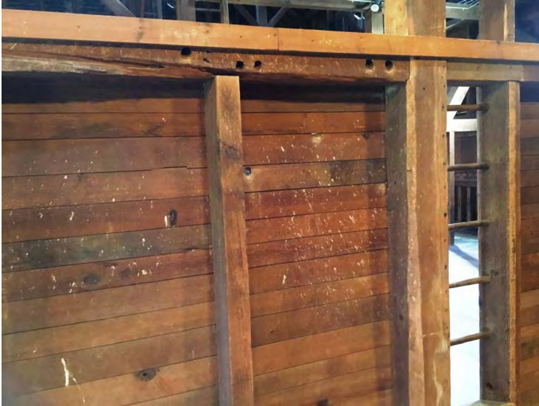
Barn interior photo 8 of 17. Mowstead wall and ladder with wicket holes in beam facing east to threshing bay
