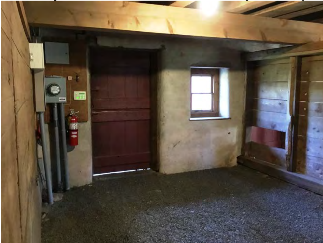
Barn interior photo 13 of 17. Stable level stall wall with wooden partition separating stall from feed aisle at right, facing south
