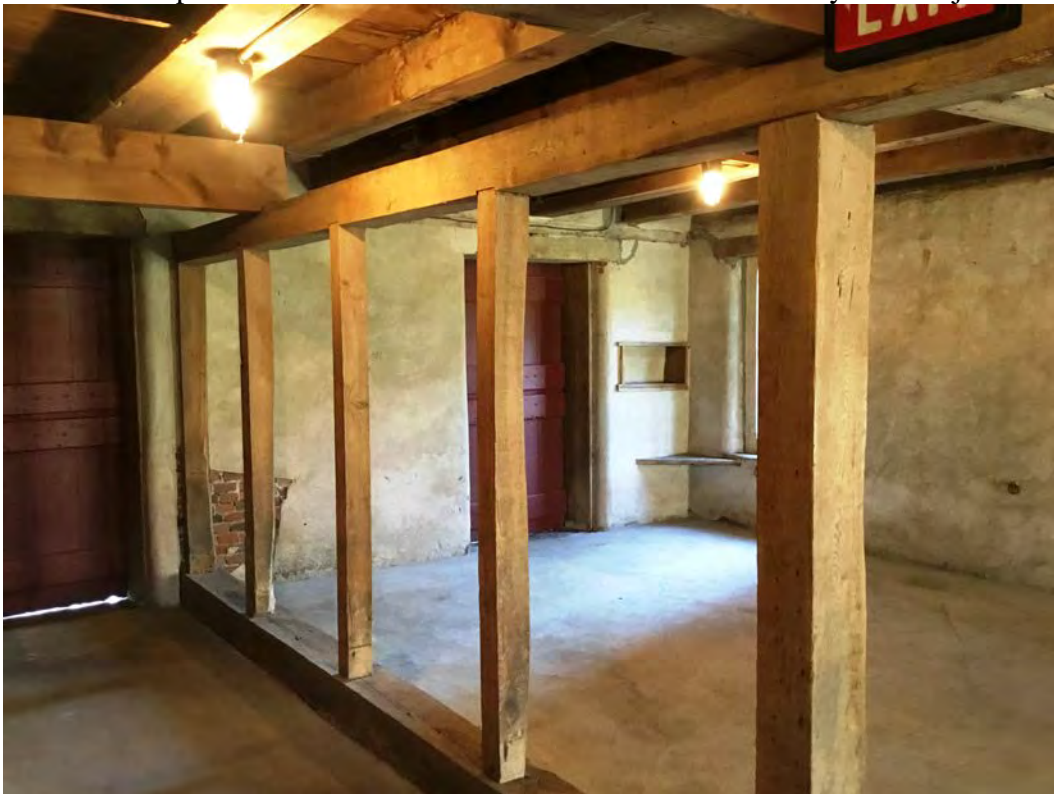
Barn interior photo 15 of 17. Stable level showing removed feed aisle wall facing southwest
