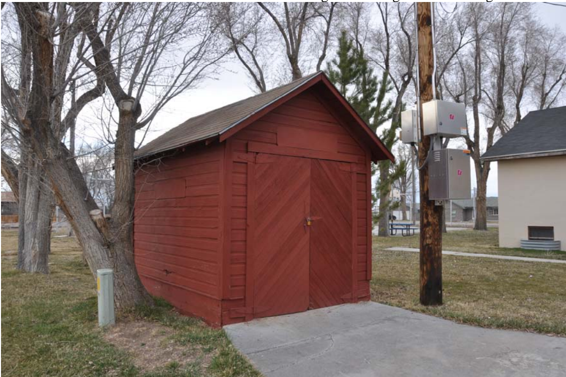
Photo No. 9. South and east elevations of non-contributing outbuilding. Camera facing northwest.
