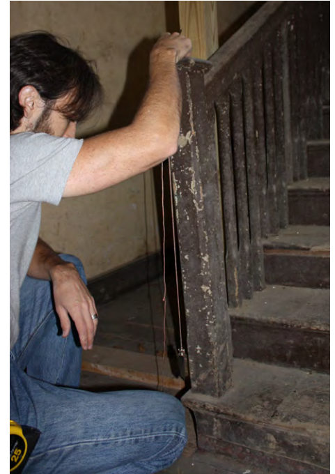
Using a plumb bob to locate the first floor newel post, Farm House
