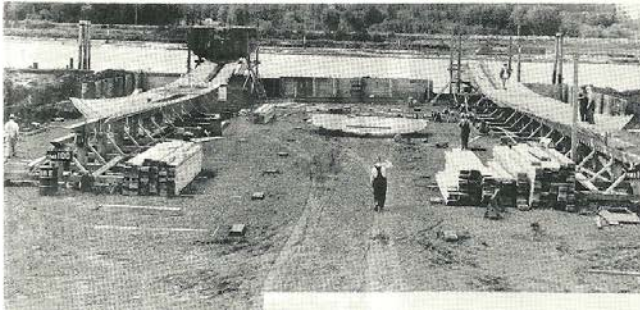
AMCCO became a war plant in late summer, 1941. The above picture shows the outdoor construction of the keels of YMS 100 and YMS 101. It was taken at 11 a.m. August 28.
