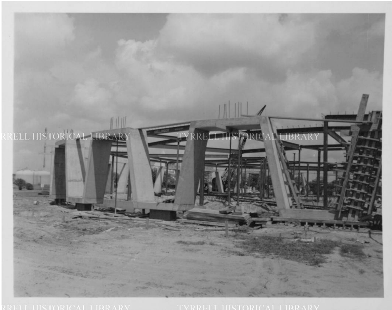
Figure 17. Construction photograph during steel framing, dated May 1959. Note on site concrete casting of perimeter “fret” band. (Dollinger Steel Company Archives at the Tyrrell Library).
