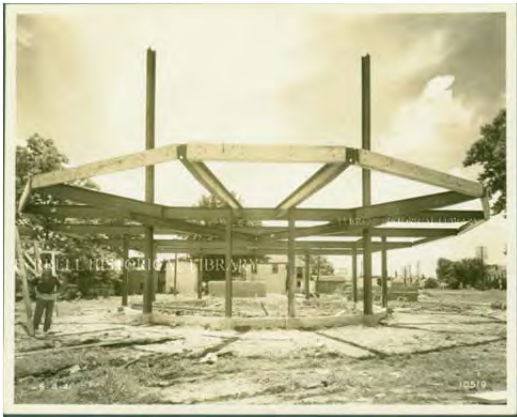
Figure 27. Pig Stand #41 steel framing by Dollinger Steel, Beaumont, Texas, c. 9/4/1941 (Dollinger Steel Company Archives at the Tyrrell Library)
