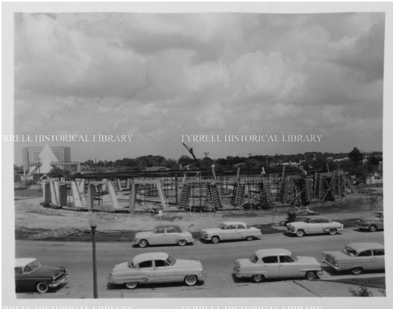
Figure 16. Construction photograph during steel framing, dated May 1959. Note on site concrete casting of perimeter "fret" band. Pyramid drive-in movie theater in background (Dollinger Steel Company Archives at the Tyrrell Library).
