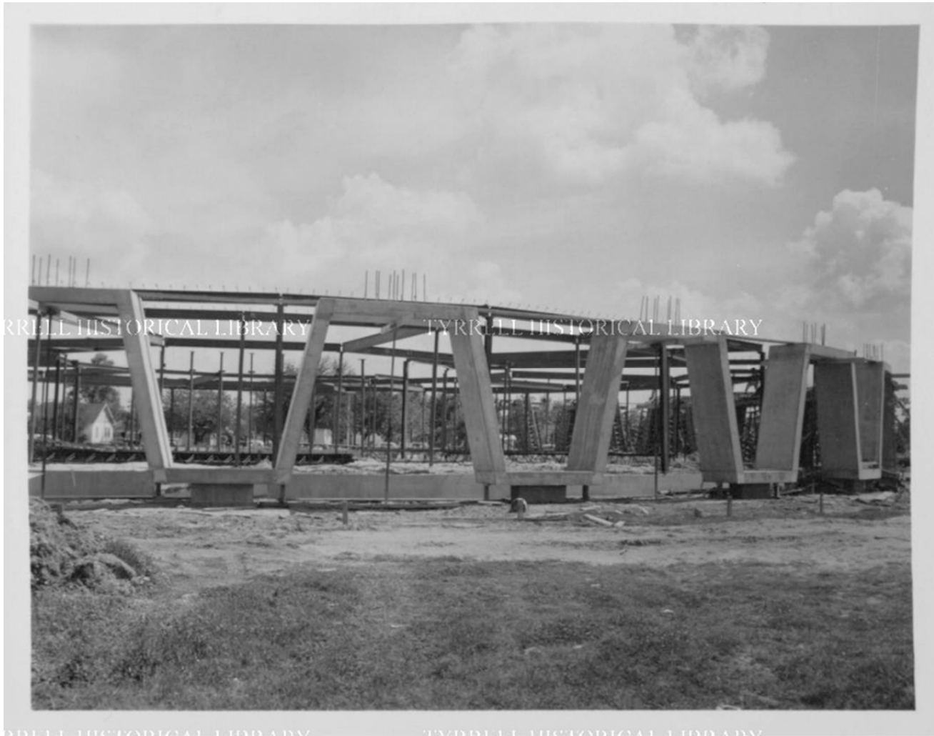
Figure 18. Construction photograph during steel framing, dated May 1959. Note exposed rebar for roof support casting. (Dollinger Steel Company Archives at the Tyrrell Library).
