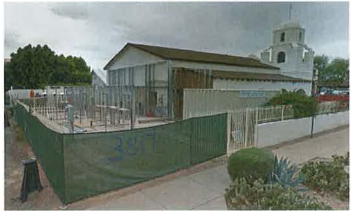
Figure 7. View facing southwest of the OLPH Mission Church during construction of the rear (east) addition showing its structural materials and connection to the original building. Source: Google, 2017.
