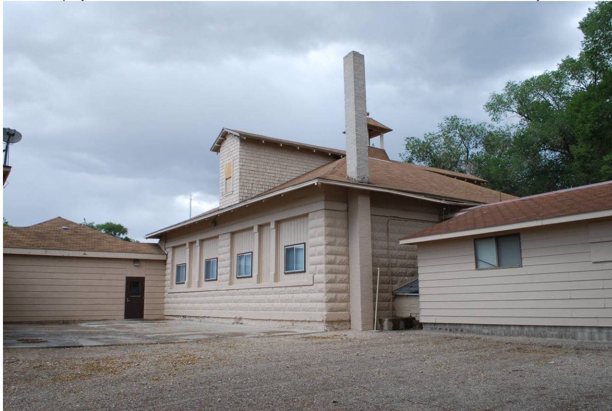
Photograph 4 – West elevation, showing chimney, Kindergarten addition (right), and class/lunchroom addition (left) (NVSHPO, 2017).
