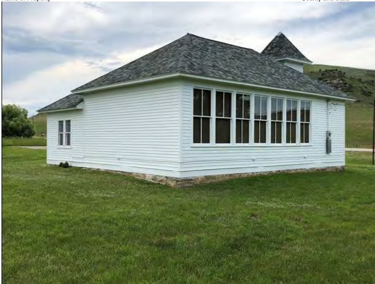
Description: Dean School, South and East elevations, view to the northwest. MT_StillwaterCounty_DeanSchool_0005
