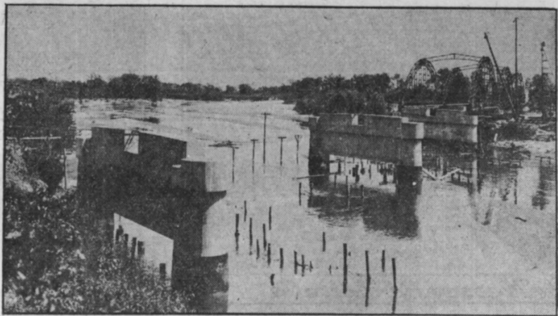
South Lawrence Avenue Bridge of Marsh Arch Design—Spanning the Arkansas River—Now Under Construction on Highway 81.
