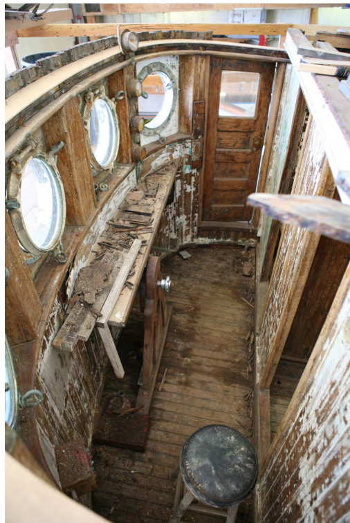
14 of 20. Western Flyer. Deckhouse, looking down into wheelhouse from scaffolding. Looking from port to starboard. Wheel has been temporarily removed during renovation.
