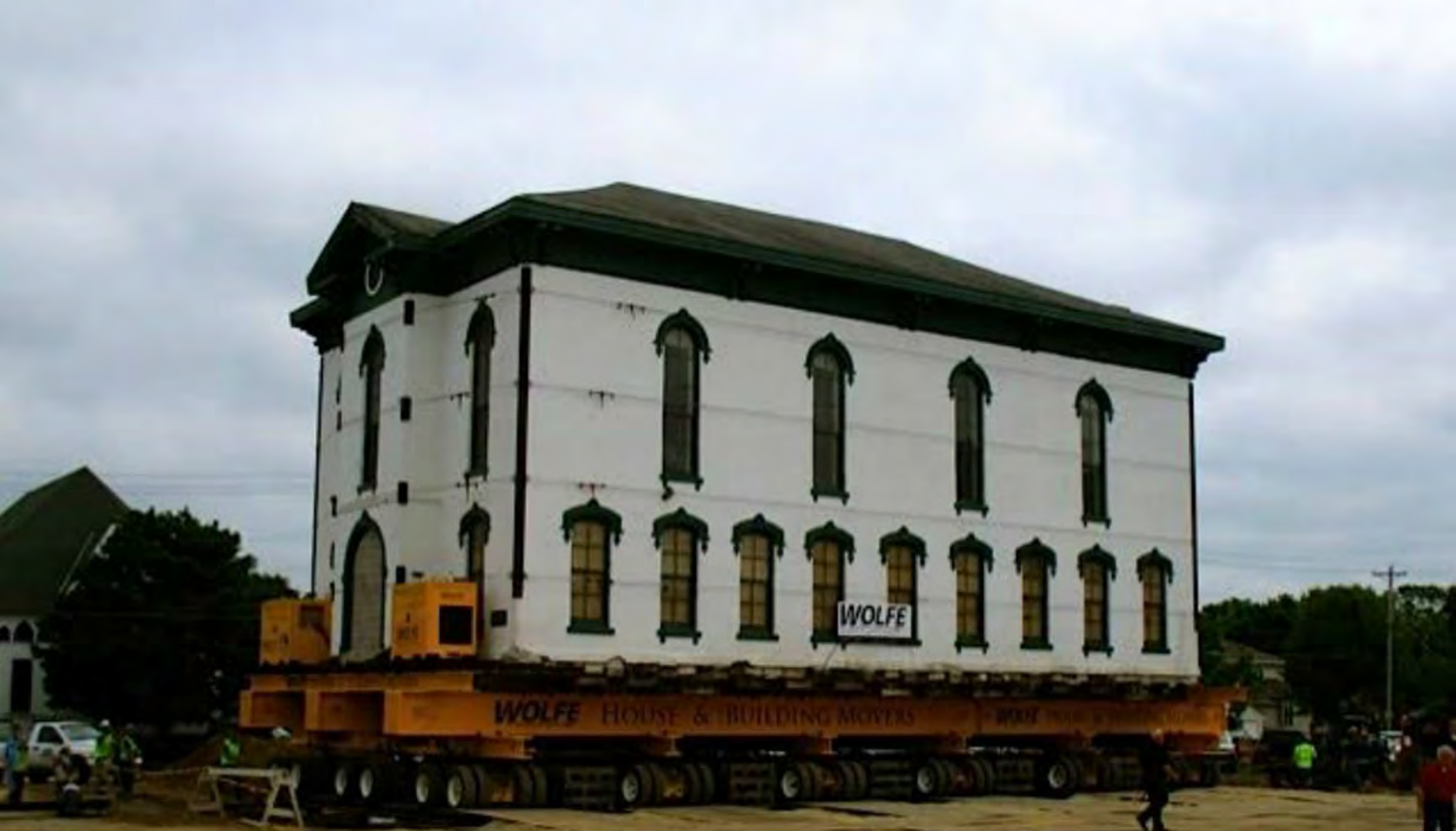
Cedar Valley Seminary Building, Osage IA, new building site, at NE corner of north 7th & Chase, building near end of move on to cribbing. Looking toward NE at front (west, original east) & south (original north) facades.
