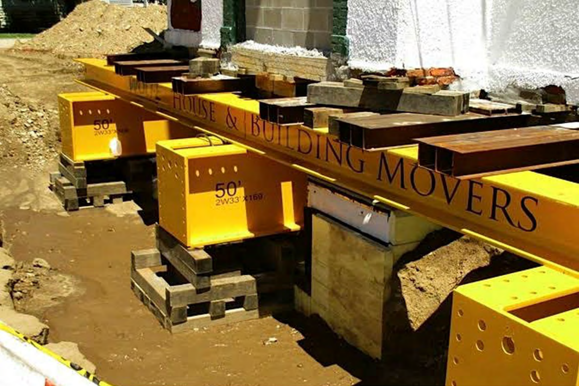
Cedar Valley Seminary Building, Osage IA, at NE corner of north 7th & Chase, close up after lowering on to cribbing. Looking toward NE at front (west, original east) facade.
