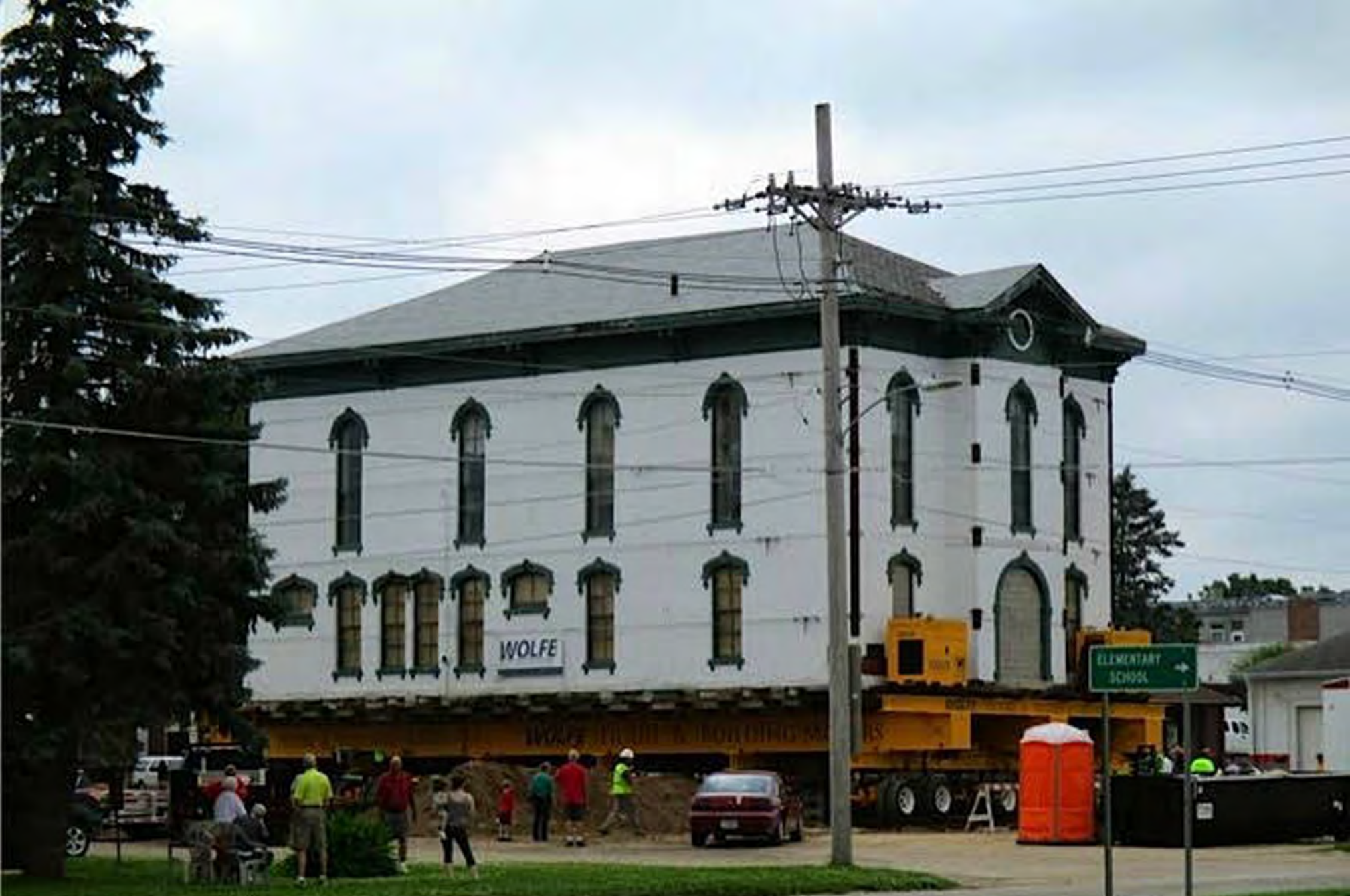
Cedar Valley Seminary Building, Osage IA, new building site, at NE corner of north 7th & Chase, at end of move on to cribbing. Looking toward SE at north (original south) &, front/west (east) facades.
