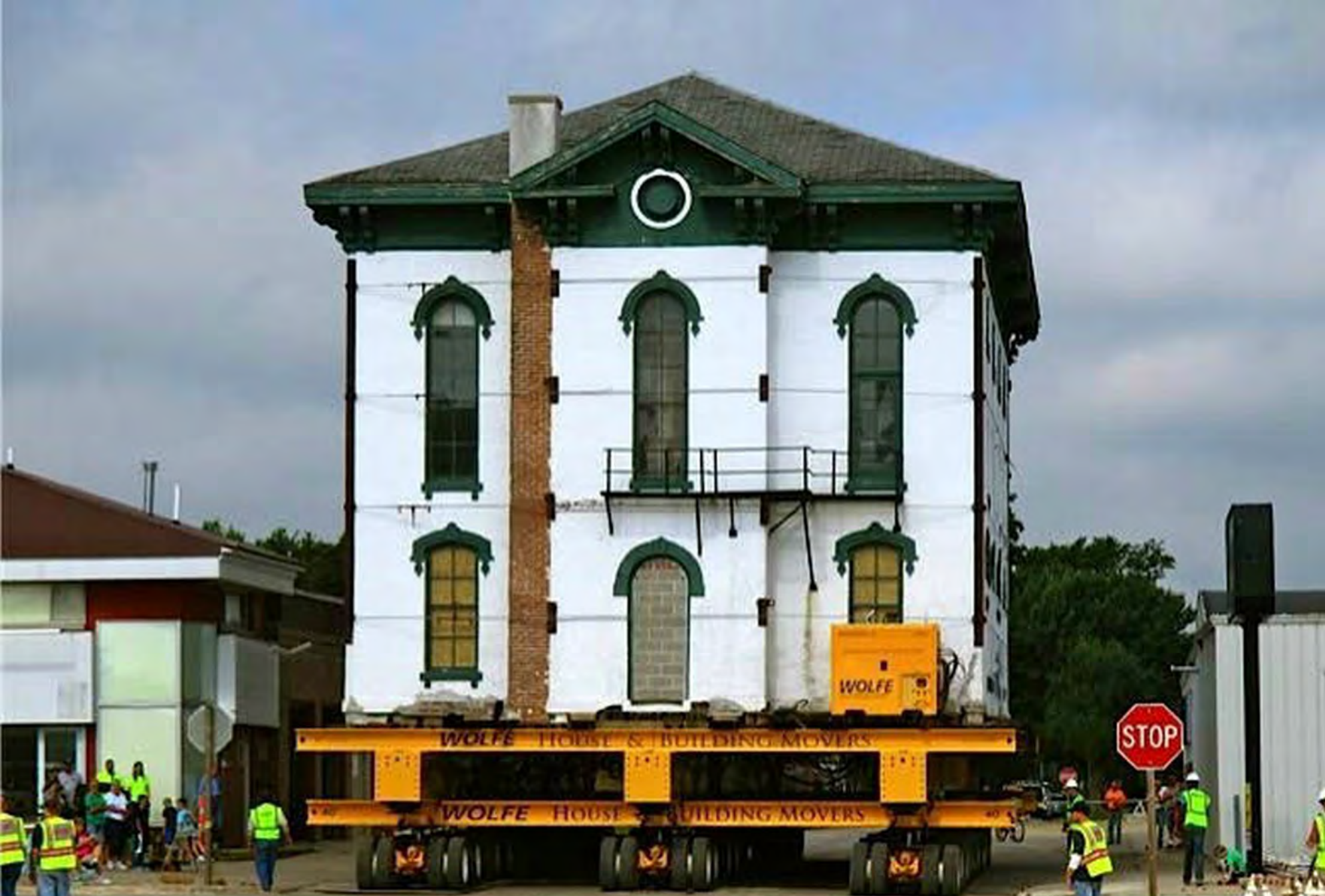
Cedar Valley Baptist Seminary Building, 1869, Osage IA, heading east at intersection of N. 7th. St & Chase Street. Entering intersection. Rear (original west) elevation.
