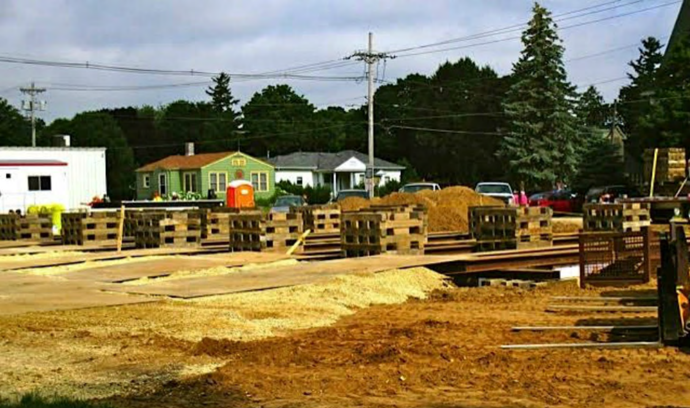
Cedar Valley Seminary Building, Osage IA, Cribbing at new building site, at NE corner of north 7th & Chase. Looking toward NW.
