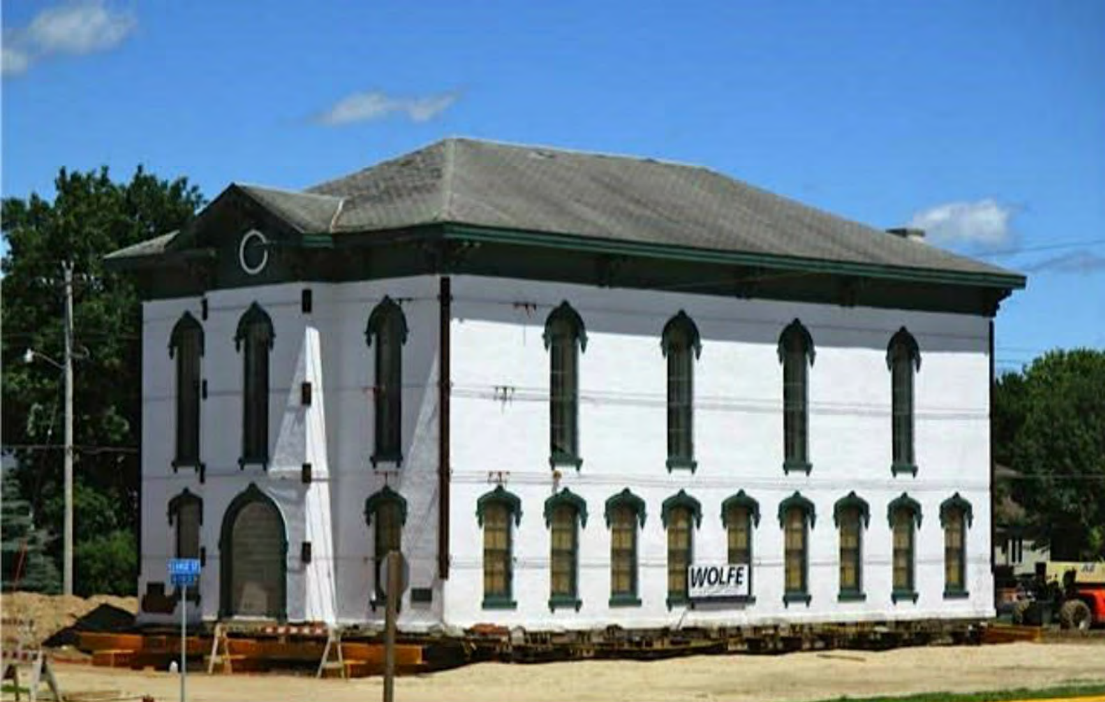
Cedar Valley Seminary Building, Osage IA, at NE corner of north 7th & Chase, building after lowering on to cribbing.
