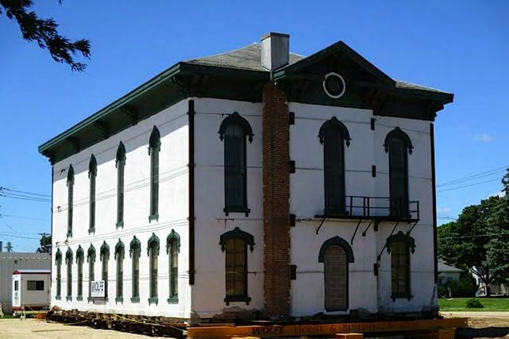
Cedar Valley Seminary Building, Osage IA, at NE corner of north 7th & Chase, building after lowering on to cribbing. Looking toward NW at rear/east (original west) & south (original north) facades.
