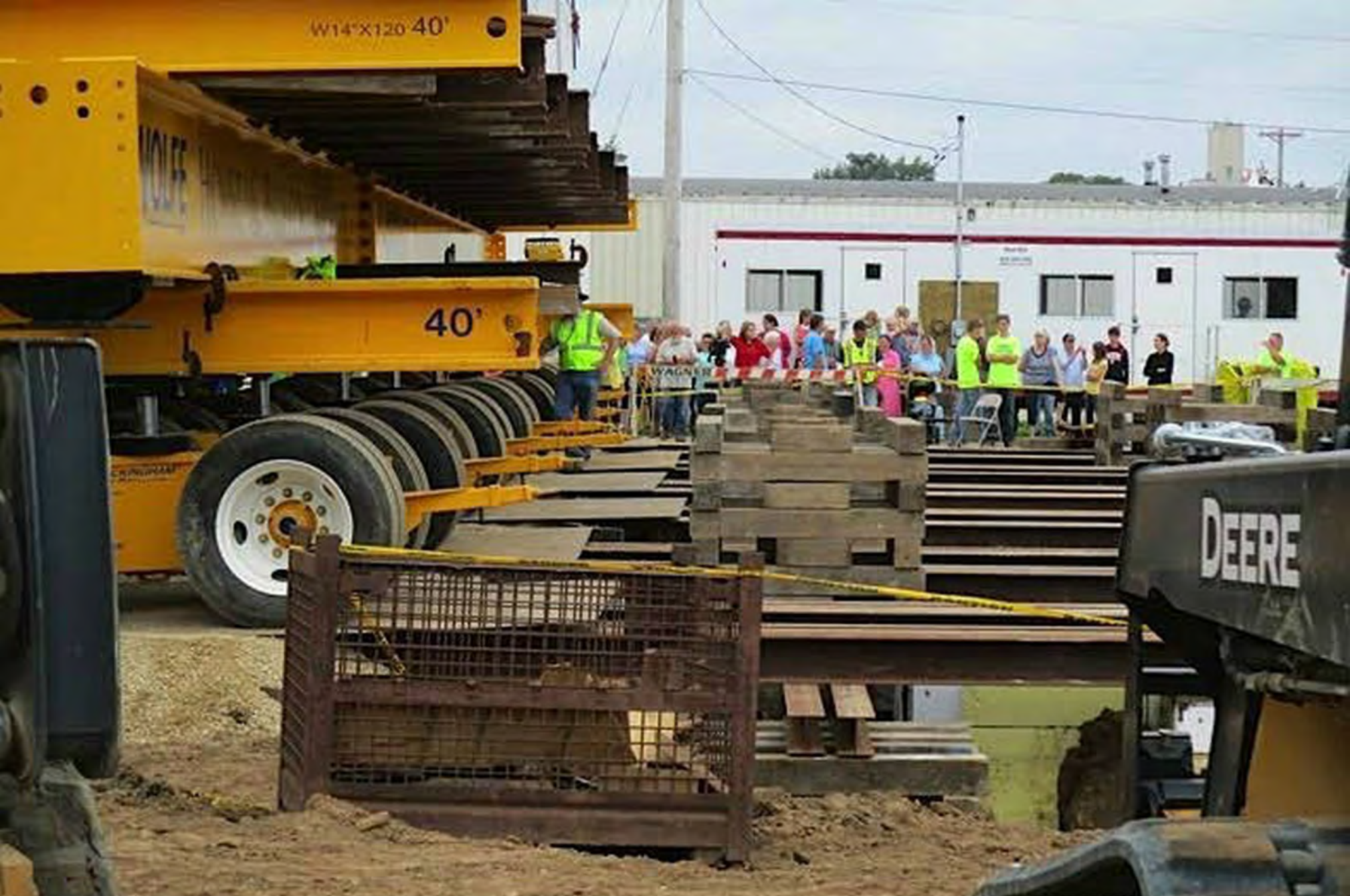
Cedar Valley Seminary Building, Osage IA, Cribbing at new building site, at NE corner of north 7th & Chase, building being moved on to cribbing. Looking west .
