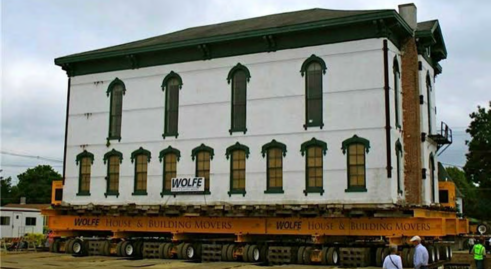
Cedar Valley Seminary Building, Osage IA, new building site, at NE corner of north 7th & Chase, building being moved on to cribbing. Looking toward NW at south (original north) facade.
