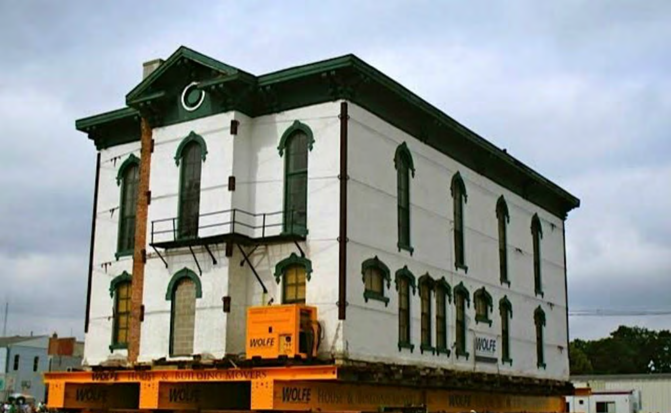
Cedar Valley Seminary Building, Osage IA, new building site, at NE corner of north 7th & Chase, Close up of building being positioned over cribbing. Looking toward west at north (original south) facade.
