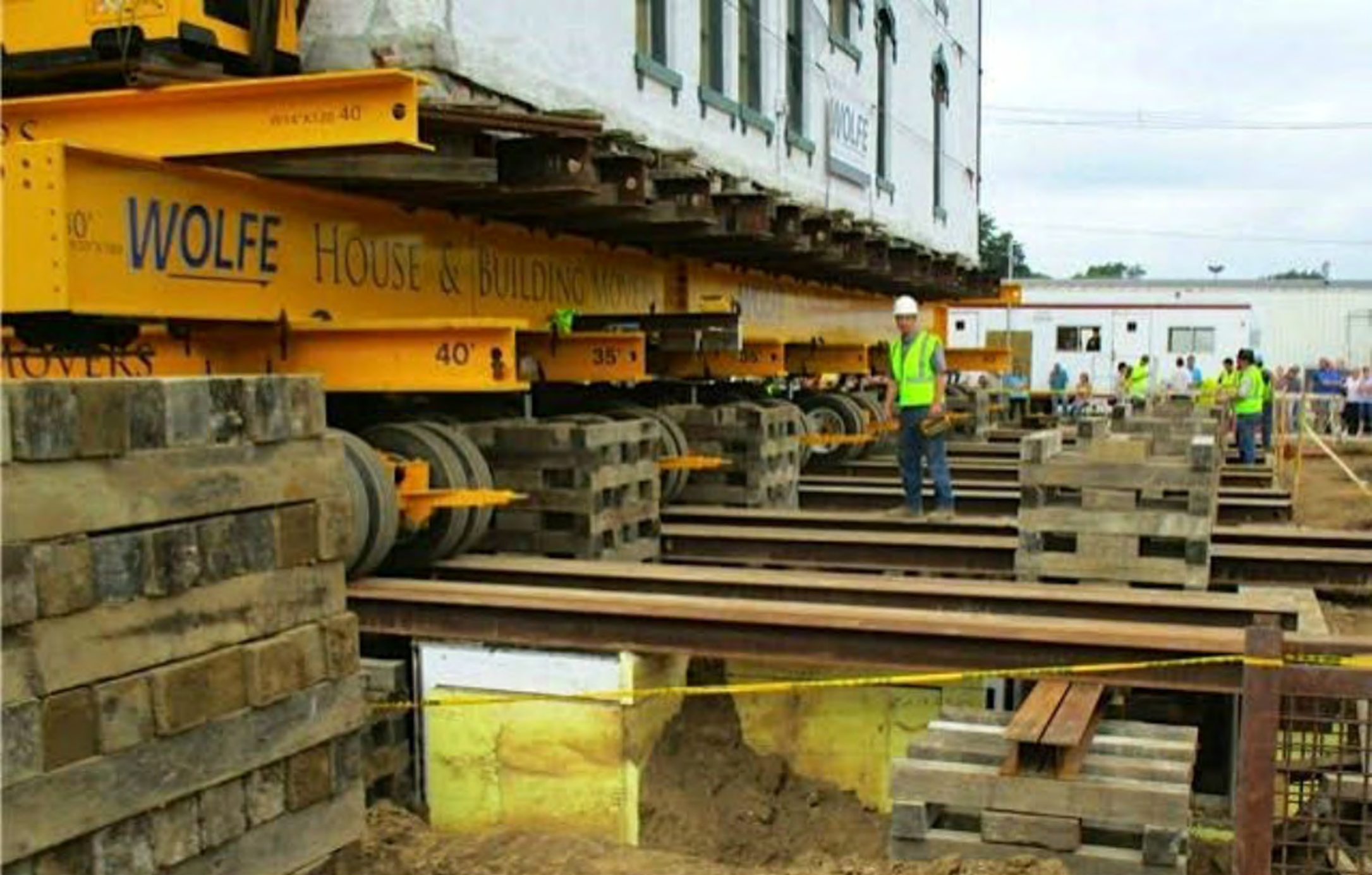
Cedar Valley Seminary Building, Osage IA, new building site, at NE corner of north 7th & Chase, Close up of building being positioned
