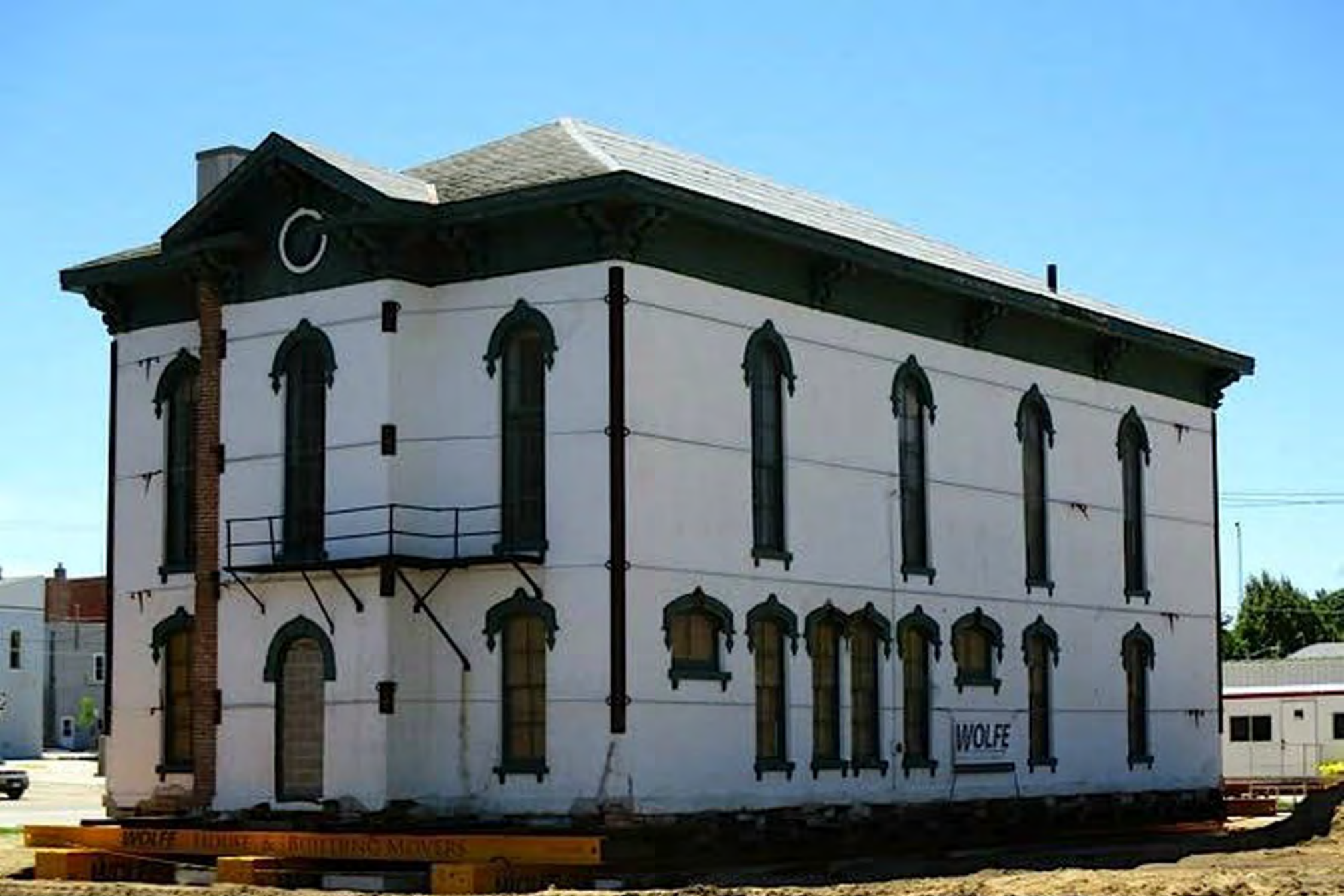
Cedar Valley Seminary Building, Osage IA, at NE corner of north 7th & Chase, building after lowering on to cribbing. Looking toward SW at rear/east (original west) & north (original south) facades.
