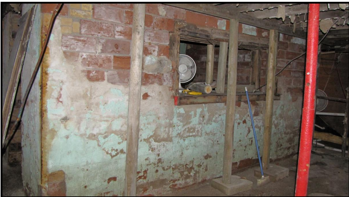
SD_Clark County_Raymond Bank_0014: Interior, basement, bank vault walls (with 'bar' cut in), view to South West.
