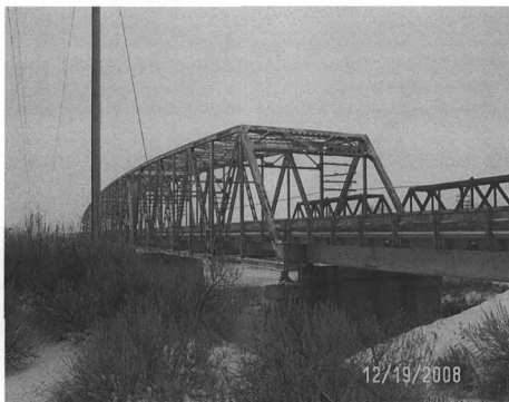
Photograph 0001. Powder River Bridge. South profile of Truss Spans. View to the northwest.
