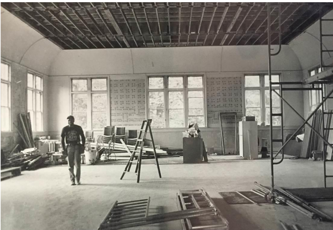
Images of renovations as the result of arson fire - c. 1992.
