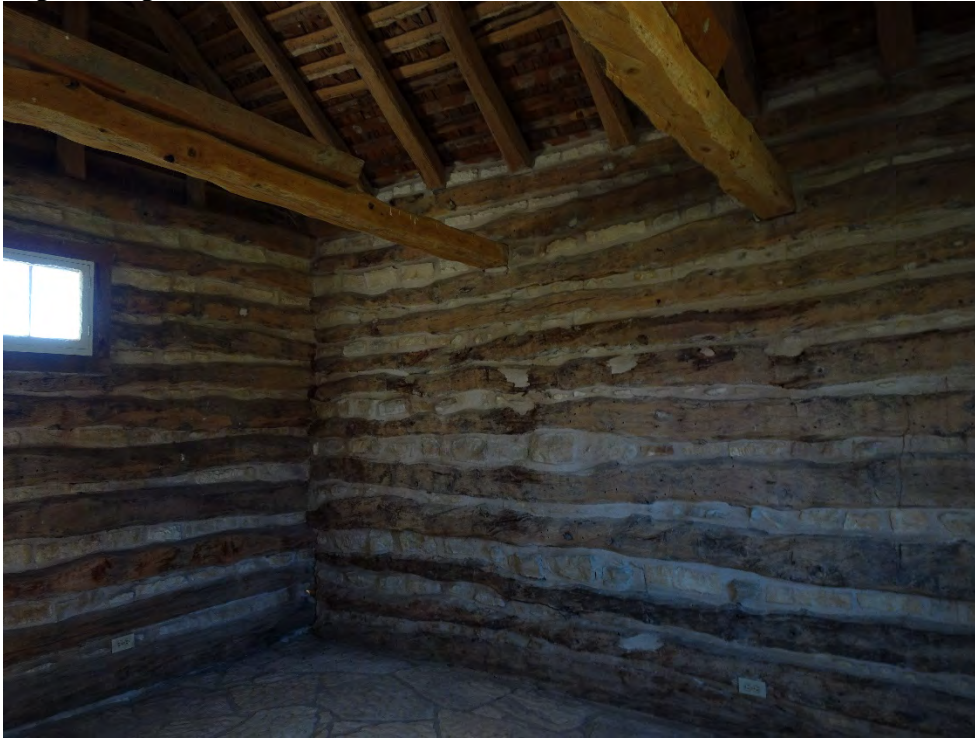
Photo 23 (TX_GillespieCounty_FellerBarsch_0023) Feller-Barsch Homestead (Resource 8) Log building. View of interior walls and roof structure.
