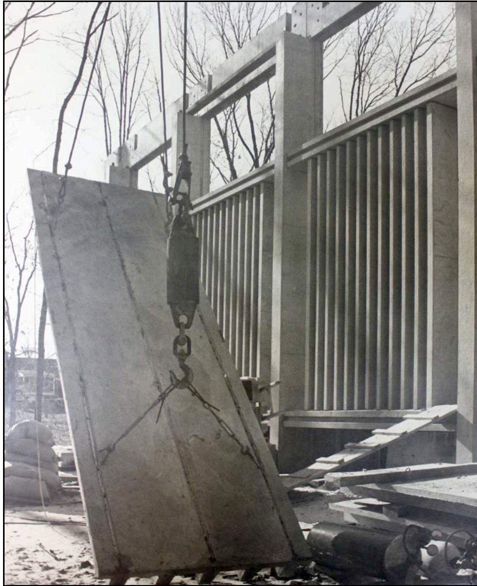
Image 24: Detail photo of Sanctuary construction, ca. 1963; photo developed June 1964 and credit to Martin Telep. From the Archives of the Unitarian Universalist Church of Arlington.
