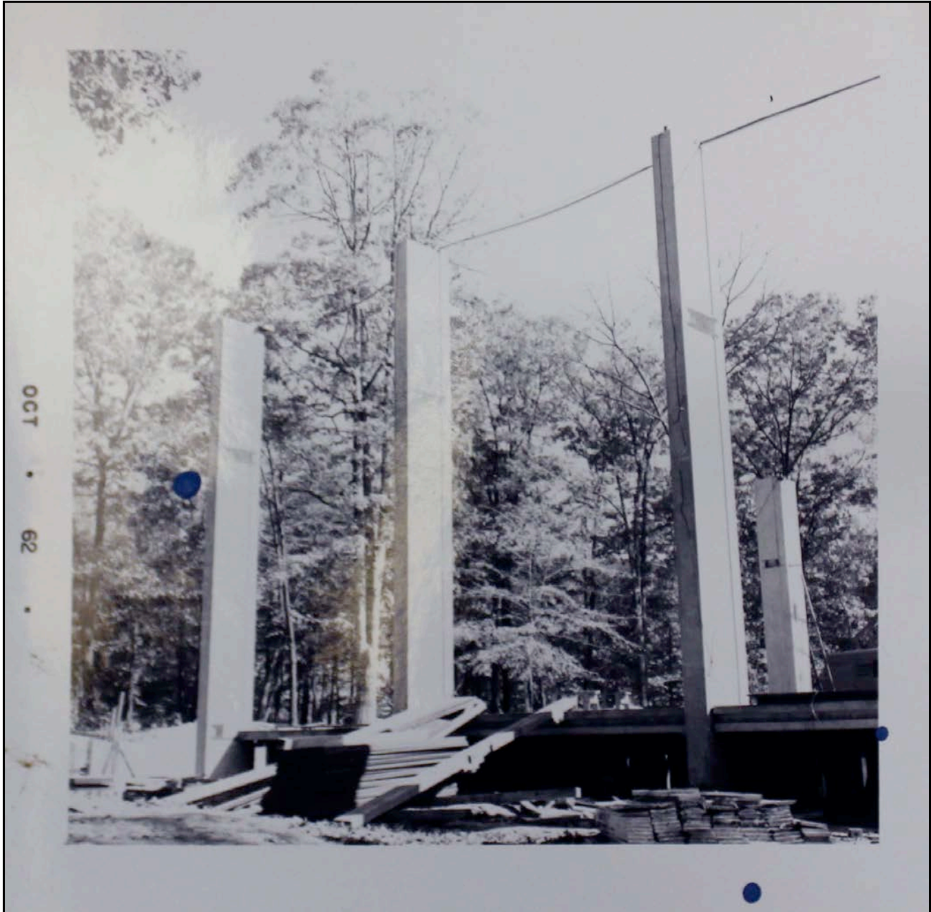
Image 22: Photo of Sanctuary Construction, dated October 1962. From the Archives of the Unitarian Universalist Church of Arlington.
