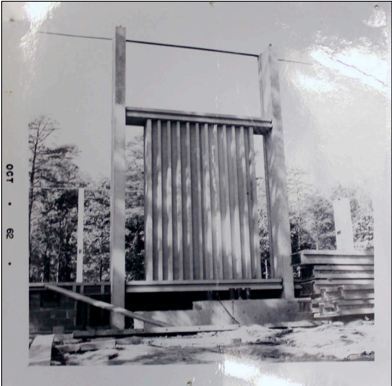
Image 23: Photo of Sanctuary Construction, detail concrete panel, dated October 1962. From the Archives of the Unitarian Universalist Church of Arlington.
