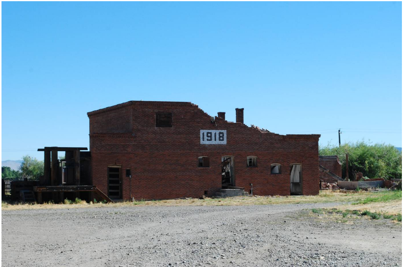
Slaughterhouse at the Dangberg Home Ranch. Built between 1915 and 1916, this was possibly the largest such facility in the region. The roof was damaged prior to 1980 but has not been repaired, leading to the current deterioration. Nevada SHPO, July 22, 2016.
