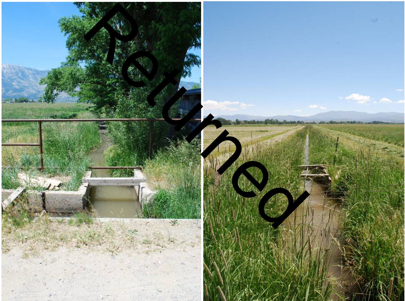
A diversion box and culvert (left) and distribution ditch (right) on the Stodieck ranches near Waterloo, Nevada SHPO, June 7, 2016.
