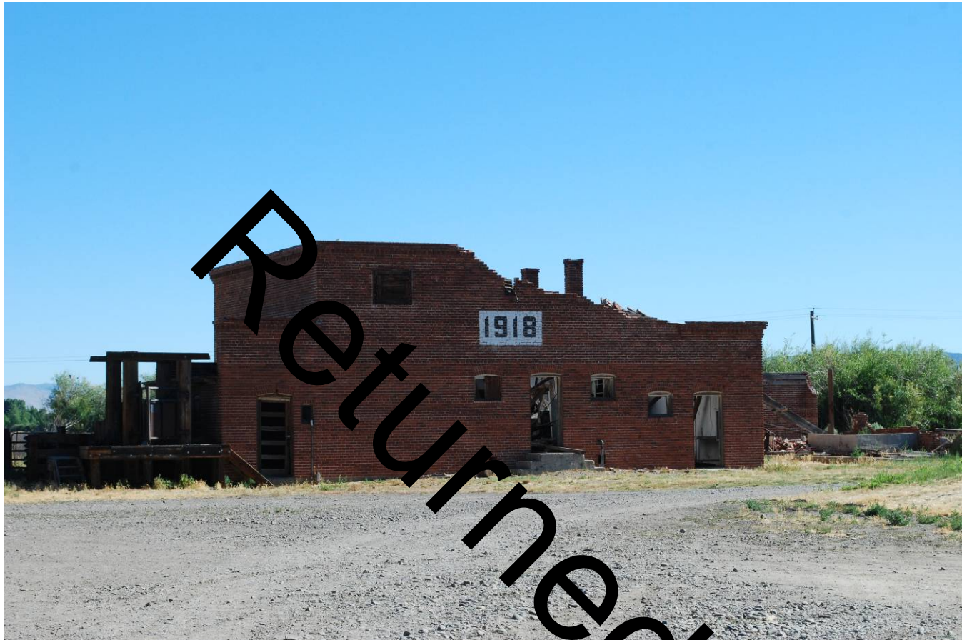
Slaughterhouse at the Dangberg Home Ranch. Built between 1915 and 1916, this is possibly the largest such facility in the region. The roof was damaged prior to 1980 but has not been repaired, leading to the current deterioration. Nevada SHPO, July 22, 2016.
