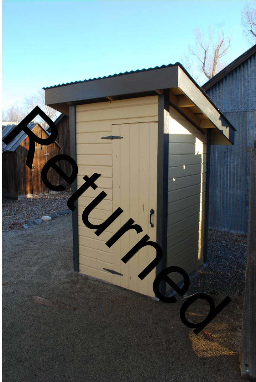
Privy at the William Lampe Ranch, constructed by the Works Progress Administration. Nevada SHPO, December 22, 2016.
