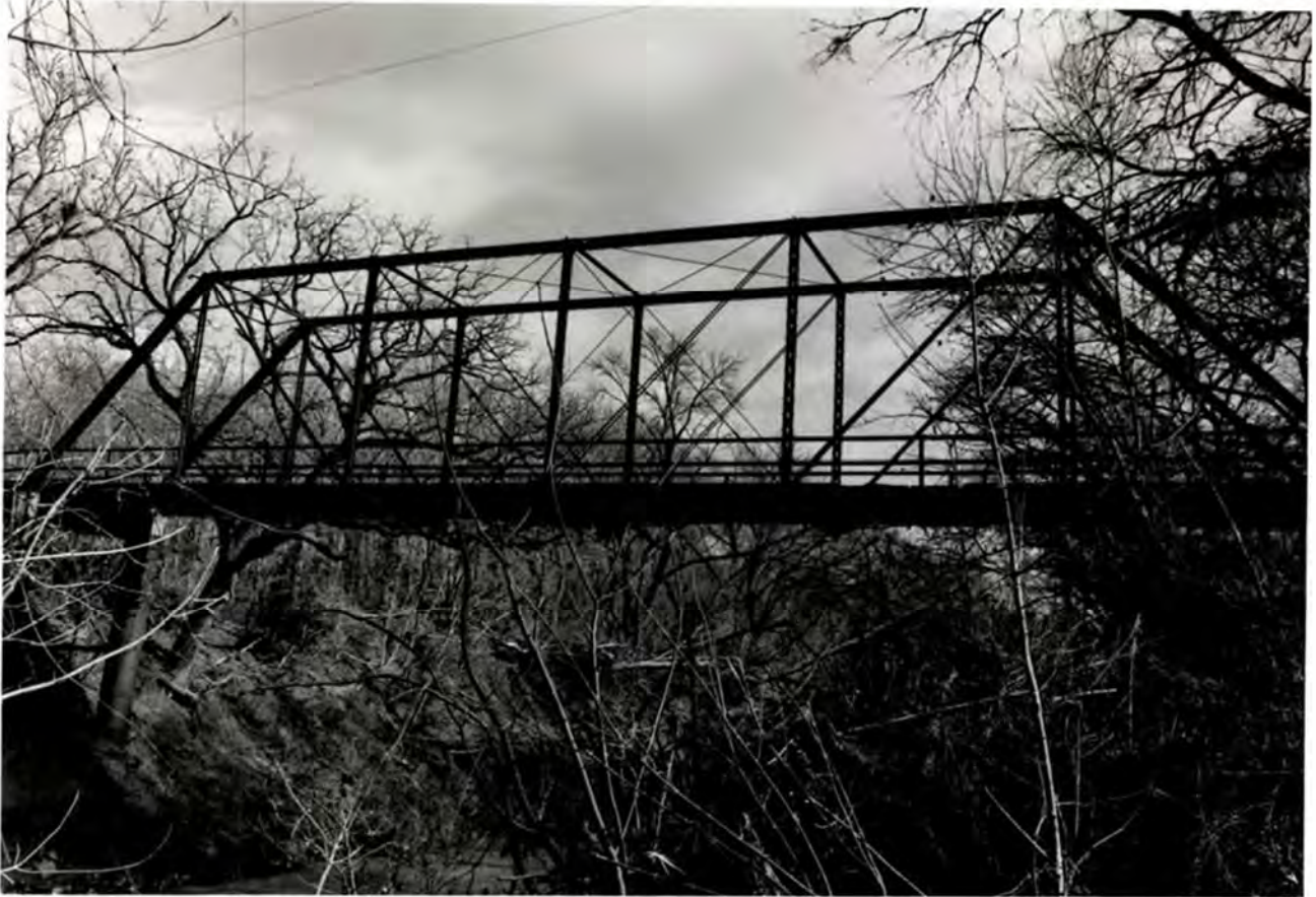
Lower Elgin Road Bridge, view east, ca. 1987 Photo courtesy Texas Department of Transportation
