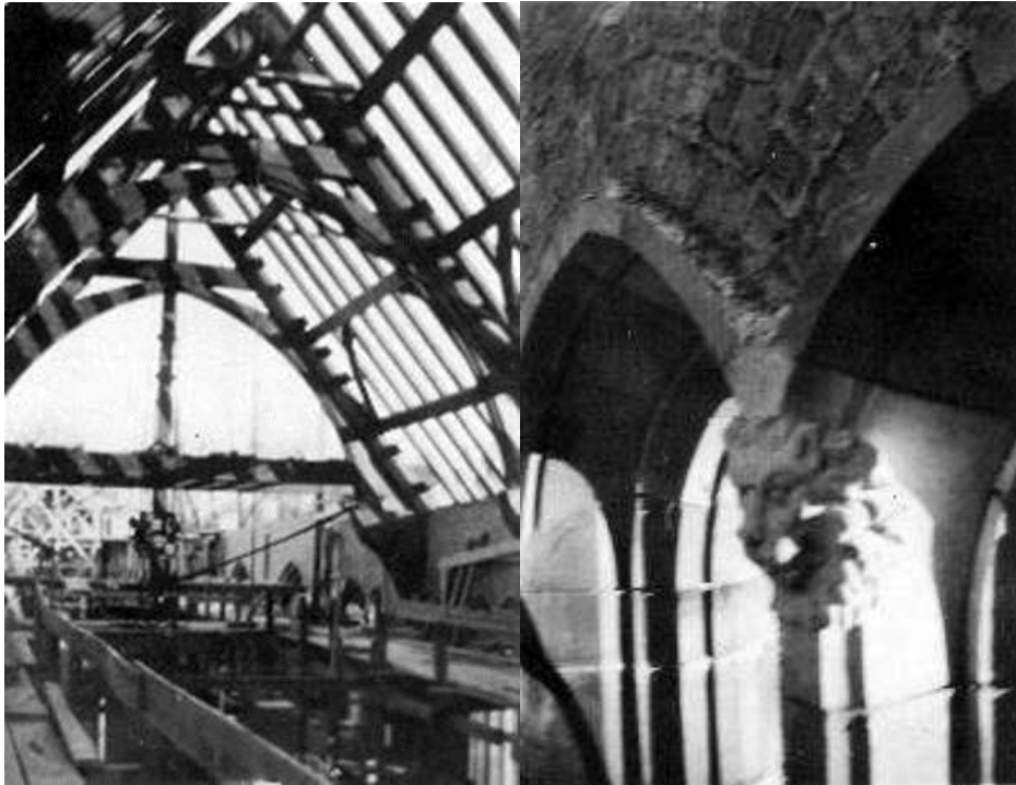
Figure 28 (left): Roof trusses, looking east, December 1925 Figure 29: Interior showing stone lion gargoyle and brickwork
