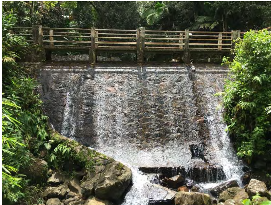
Figure 5. View of the masonry dam and elevated concrete walkway (towards the west).
