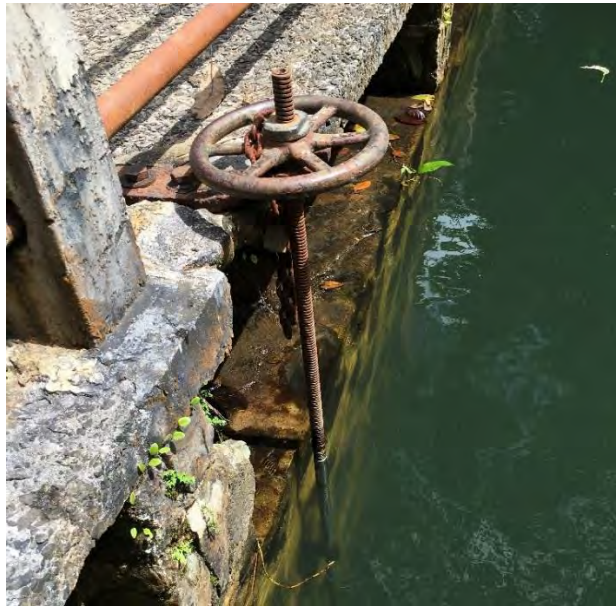
Figure 6. Sluiceway valve (towards the southeast)
