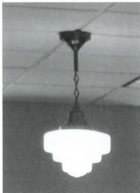
Figure 9: Original light fixture in computer lab. Camera facing east.
