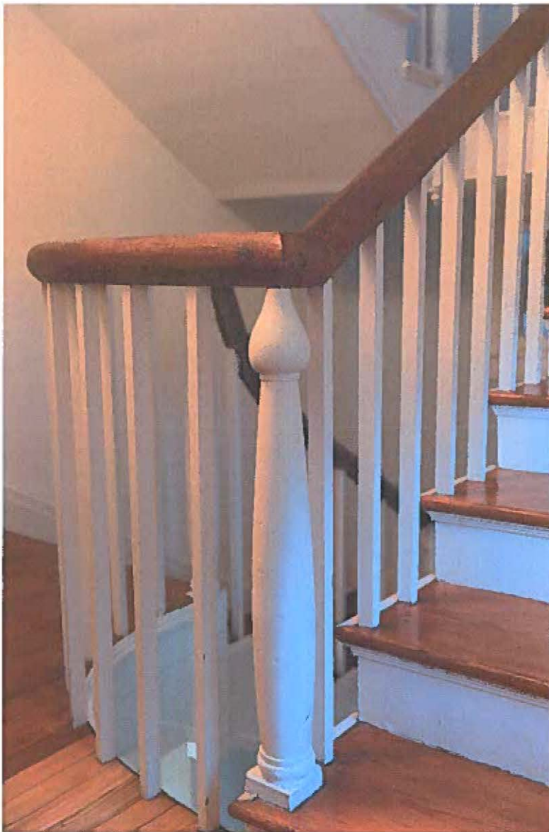
MD_FrederickCounty_Cockey'sHouseandStore_0026.tif Cockey/Jamison/Hendrickson House interior, second floor stairway landing, banister and newel post
