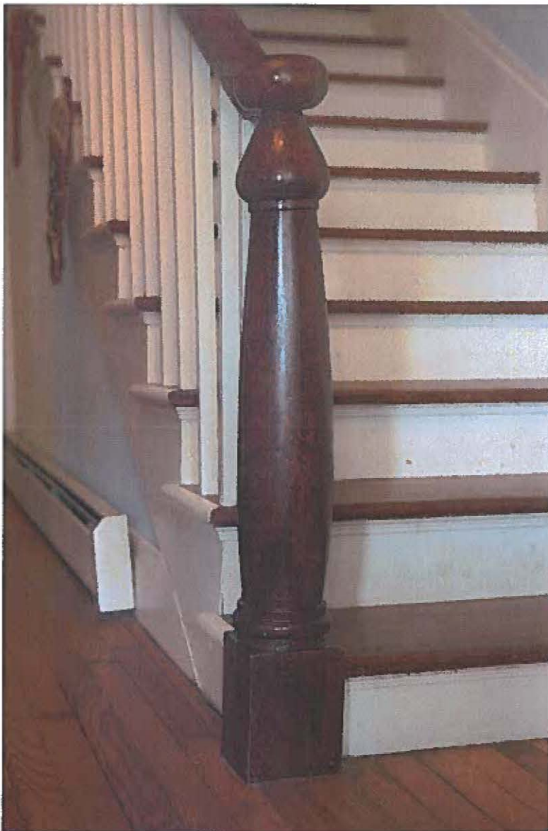
MD_FrederickCounty_Cockey'sHouseandStore_0017.tif Cockey/Jamison/Hendrickson House interior, front hall stairway, newel post of solid walnut
