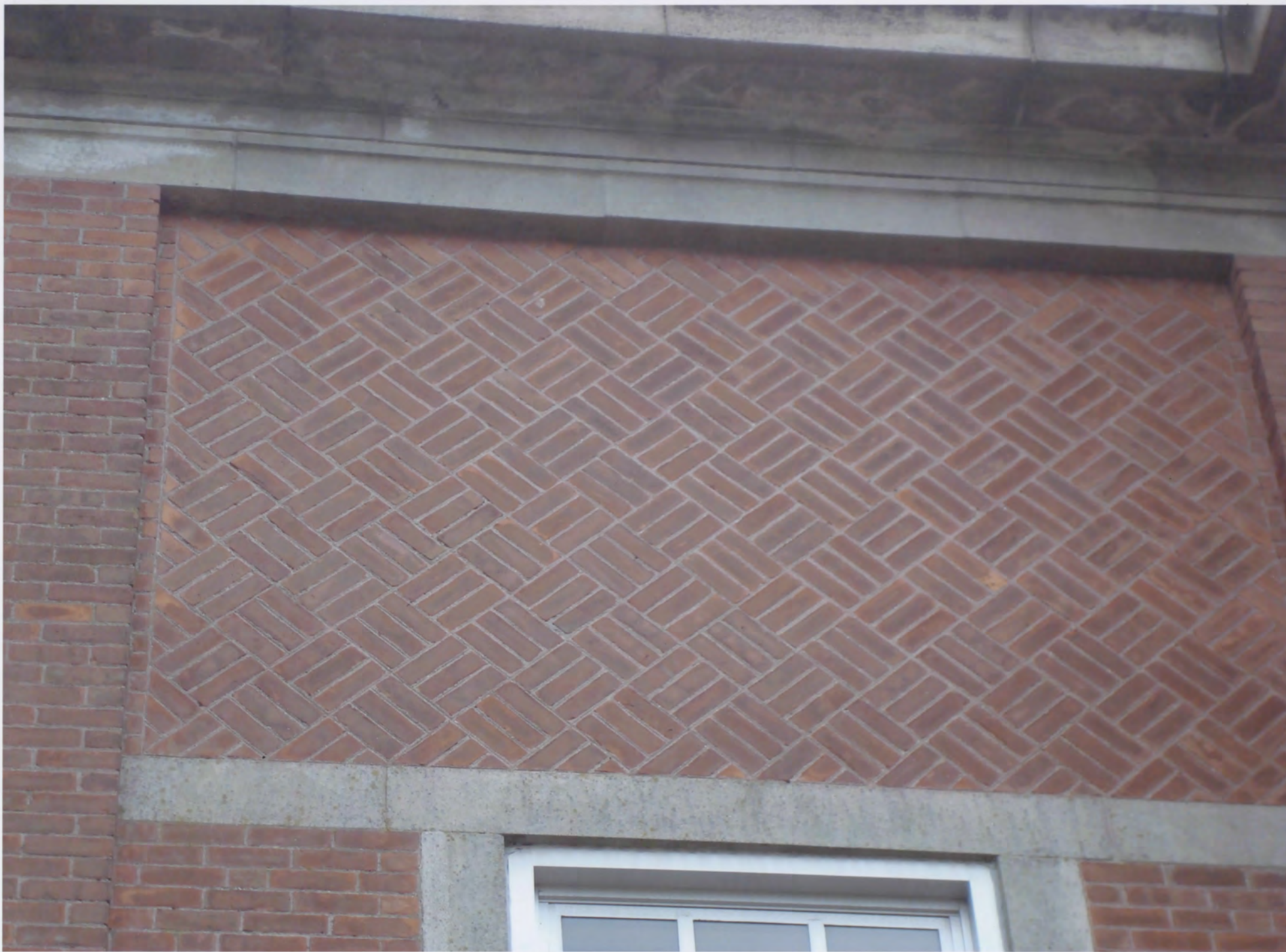
6. North elevation detail showing basket weave brick panel (Photographer: Jennifer M. Goldson, 2010)
