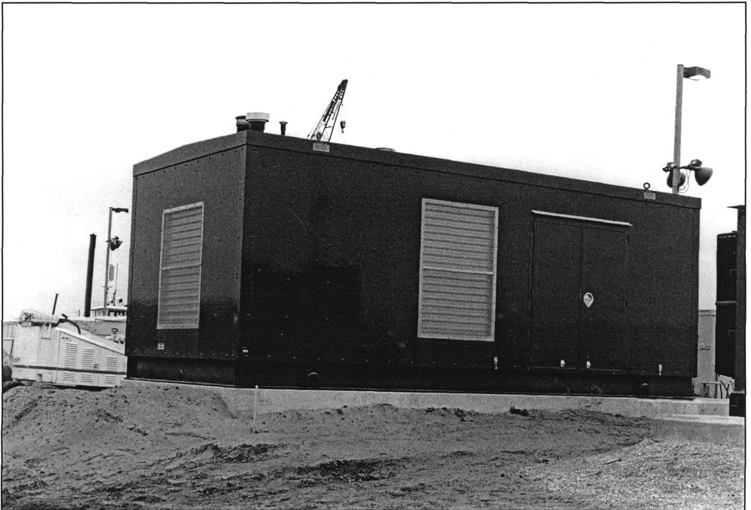
PHOTO 9. Generator. Photographer: Date of Photograph: Location of Original Negative:
