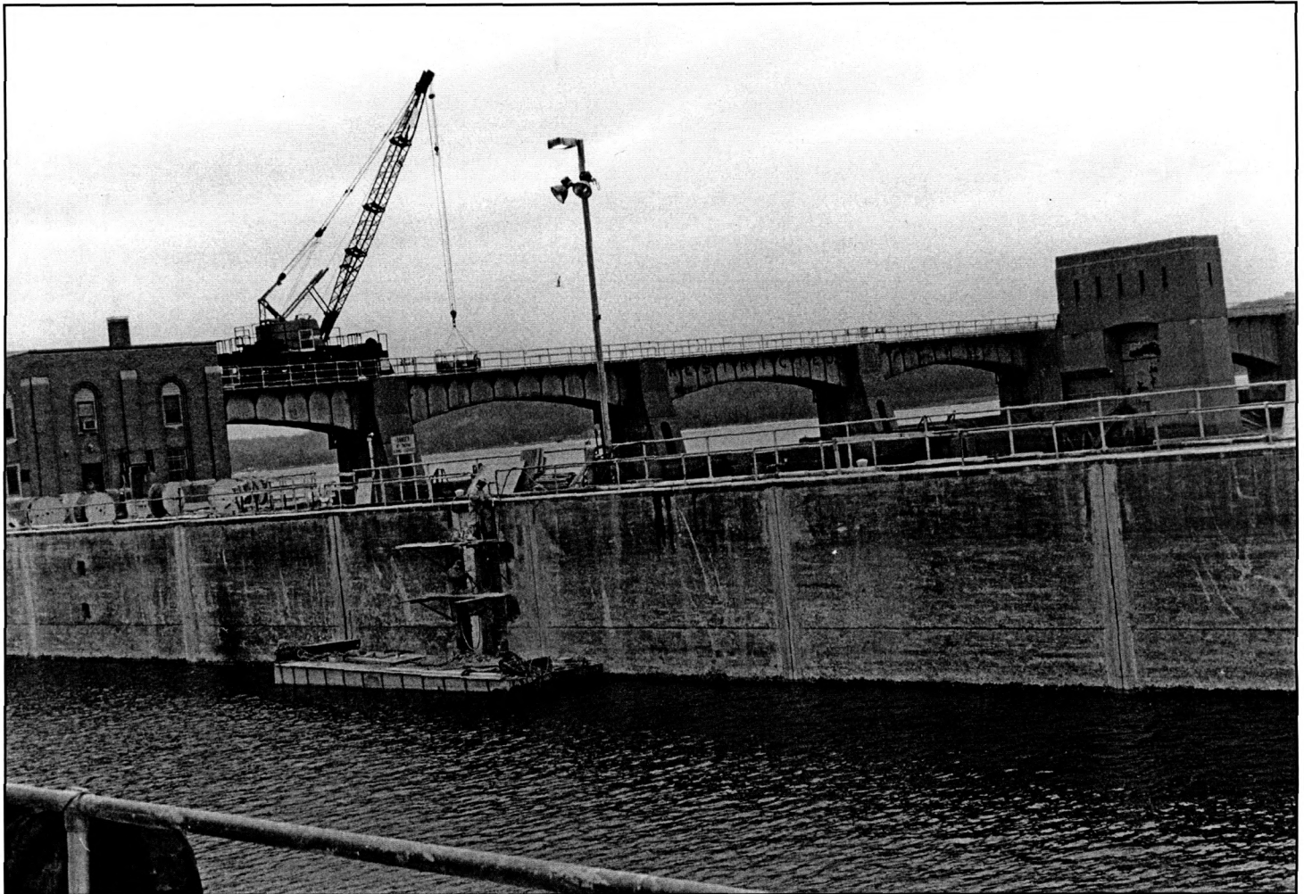
PHOTO 3. Men Working on Rehabilitation of Lockward Face of South Wall of Main Lock. Photographer: Mary Yeater Rathbun Date of Photograph: February 1998 Location of Original Negative: URM-NATIONAL REGISTER, roll #2, frame 22, Environmental Impact Section, Planning Division, Rock Island District, U.S. Army Corps of Engineers, Rock Island, IL. View: From downstream end of land wall of lock, looking northeast
