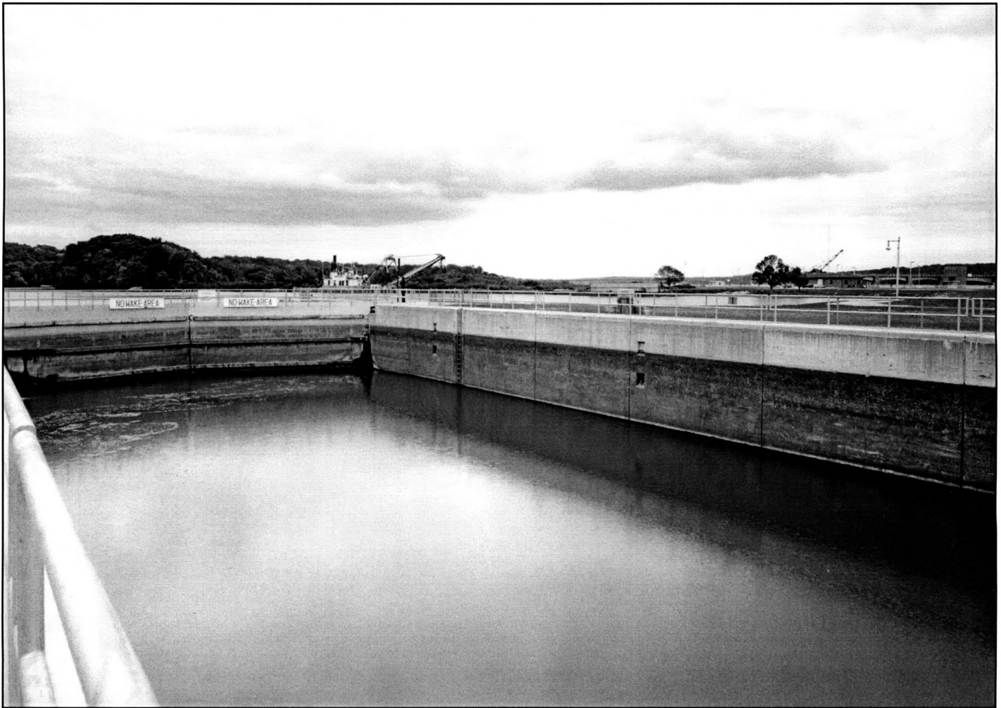
PHOTO 5. General View of Old Le Claire Lock, Downstream Side of Upstream Gates and Lockward Face of East (Riverward) Lock Wall. Photographer: Peter A. Rathbun Date of Photograph: September 1987 Location of Original Negative: IA-25-20, HAER, IOWA, 82-LECLA.V,1-HAER Collection, Prints and Photographs Division, Library of Congress, Washington, D.C. View: From land wall of lock, looking northeast
