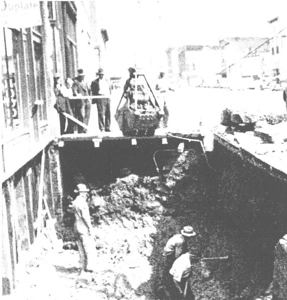
PHOTO No. 17—1937 PHOTOGRAPH OF EXCAVATION BELOW THE SIDEWALK IN FRONT OF THE MORSE HARDWARE COMPANY BUILDING TO EXTEND THE BASEMENT. SOURCE: SELL'EM LOW—SEND AND GET MORE: A CENTENNIAL HISTORY OF THE MORSE HARDWARE COMPANY, 1884-1984: 59.
