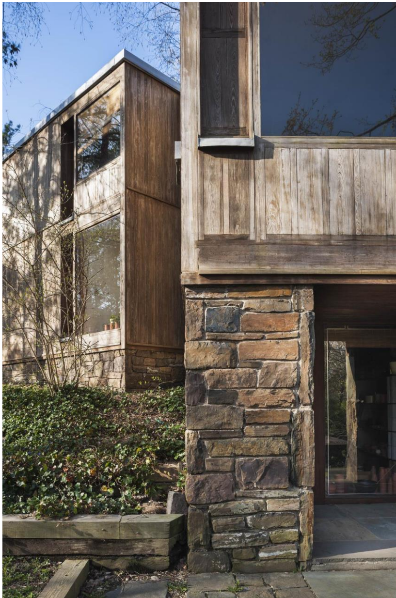
Photo 5 – Detail view of northeast elevation, showing the bottom of a deeply-inset window unit lined with a lead-coated copper drip pan. Below, an opening in the Montgomeryville stone foundation leads to the ground-level basement area.
