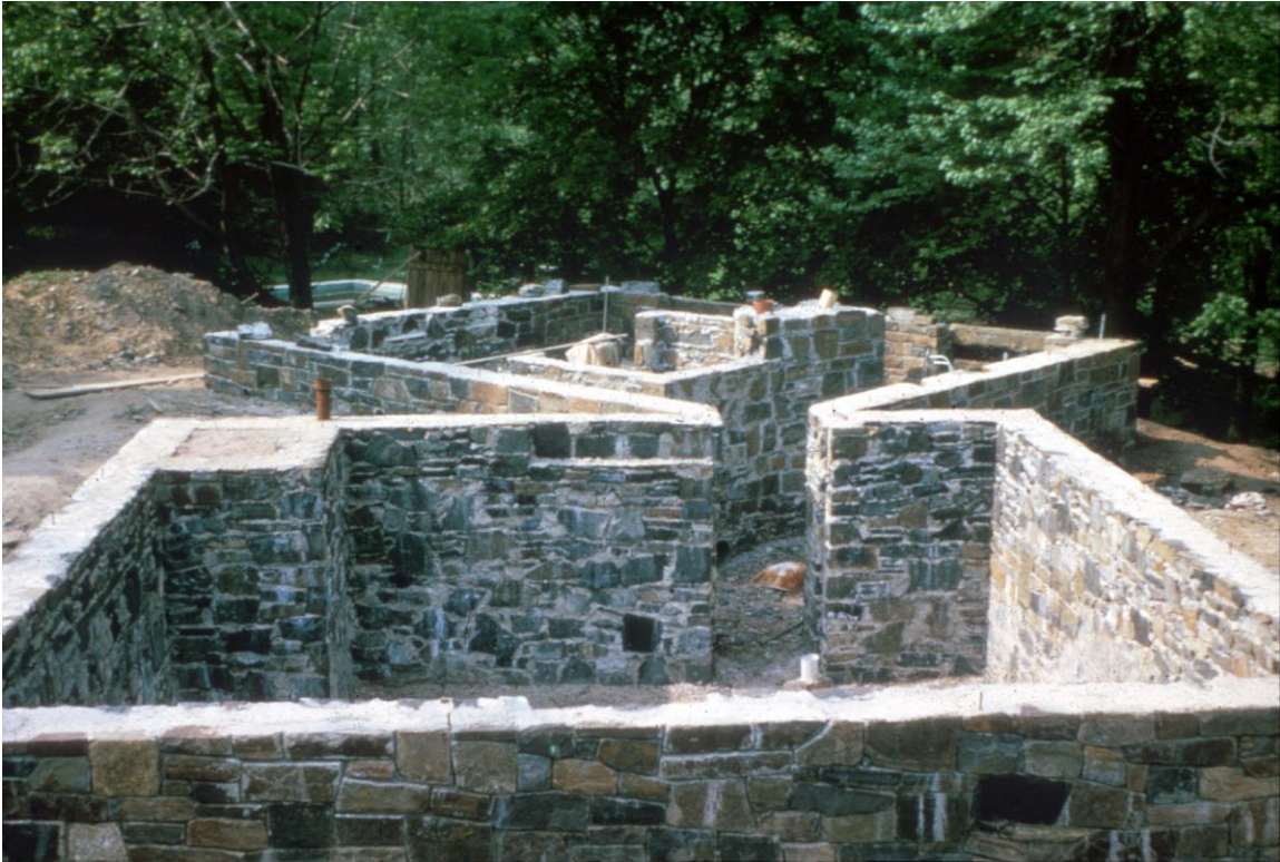
Photo 22 – This image from 1965 shows the one-story stone foundation during construction. Kahn had a vision for the monumental foundation and made at least five trips to the site to inspect and ensure its proper execution. (Norman Fisher, Photographer, courtesy of The Architectural Archives, University of Pennsylvania by the gift of Norman and Doris Fisher)
