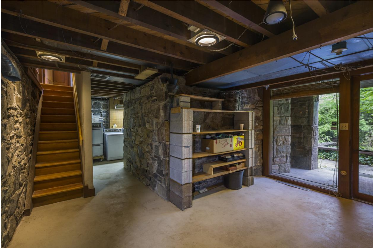
Photo 20 - Composed of several simple, open spaces enclosed by the stone foundation walls, the basement's primary functions are to house mechanical functions, the laundry, storage, and a workshop space. (National Trust/Tom Crane, Photographer)
