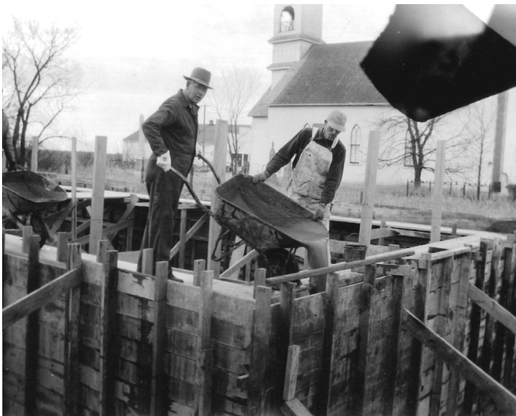
c. Placing concrete mix within board form foundation walls; church is in background
