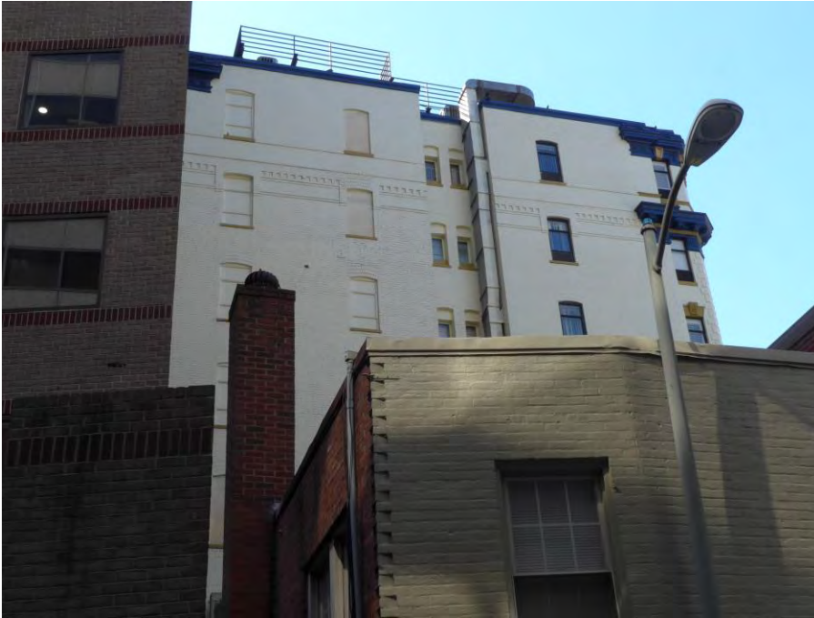
View looking west (skyward) showing east elevation at upper level Photo 10 of 17
