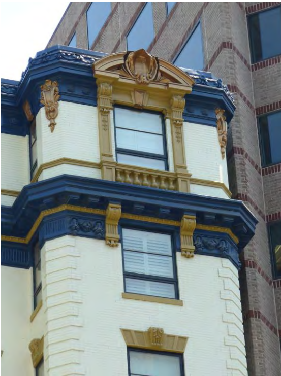
Exterior detail of south end of west elevation at attic level Photo 7 of 17
