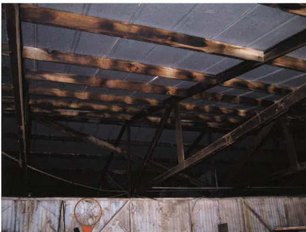
Photograph 9. Barn trusses, showing scorching from 1935 fire, facing southeast.
