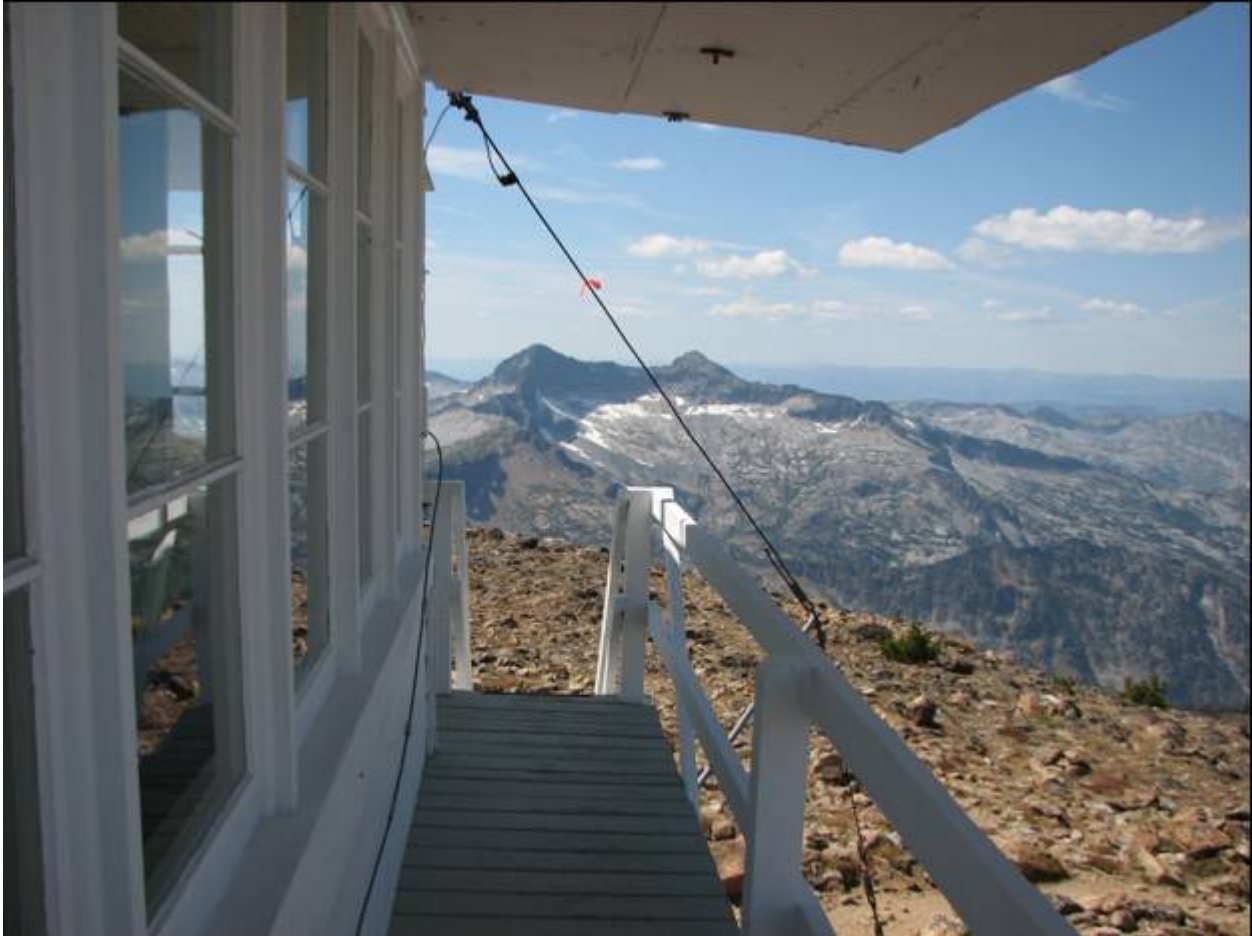
MT_RavalliCounty_StMaryPeakLookout_0004. Looking west along the north side of the catwalk to the stairway.
