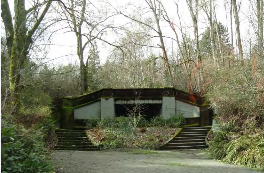
Photo 14. WA_KingCounty_LakeWashingtonBoulevard_0014. Colman Park Overpass No. 1 (contributing resource no. 4) in Colman Park carries Lake Washington Boulevard, view west.
