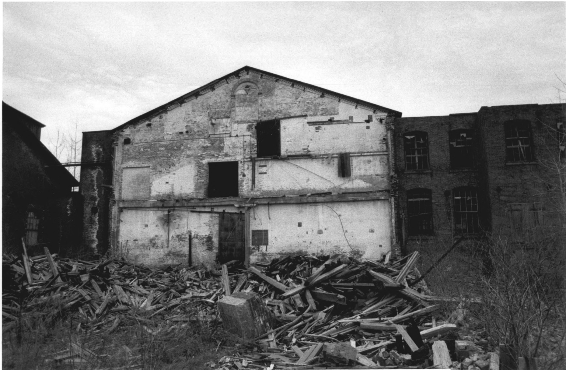
Photo 13: New Power Mill, West End, with partially demolished adjacent building at right.
