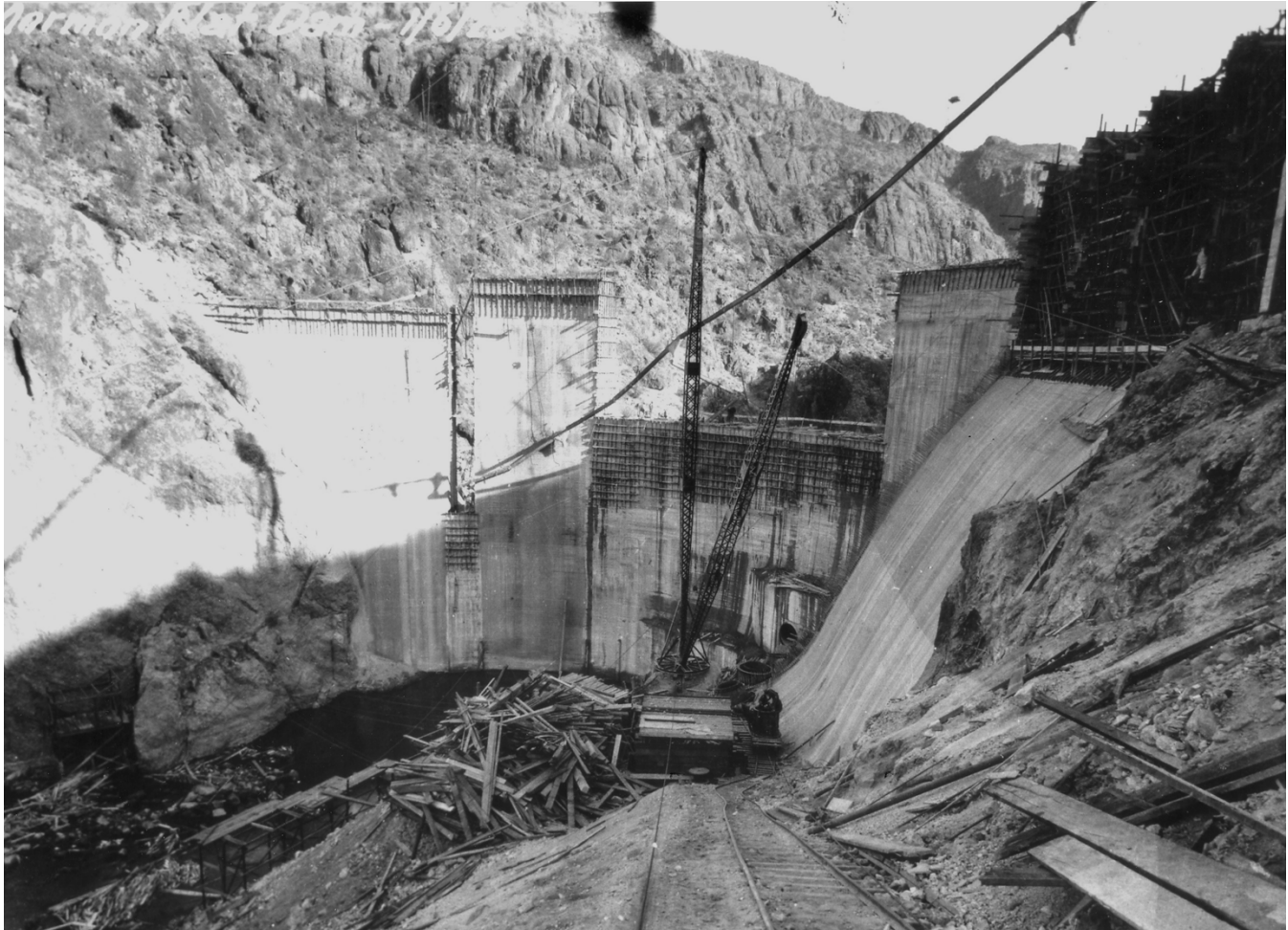
Historic Photo 6: View of downstream face showing section being keyed, January 1925. Spillway apron is at right. Photo courtesy of the SRP.
