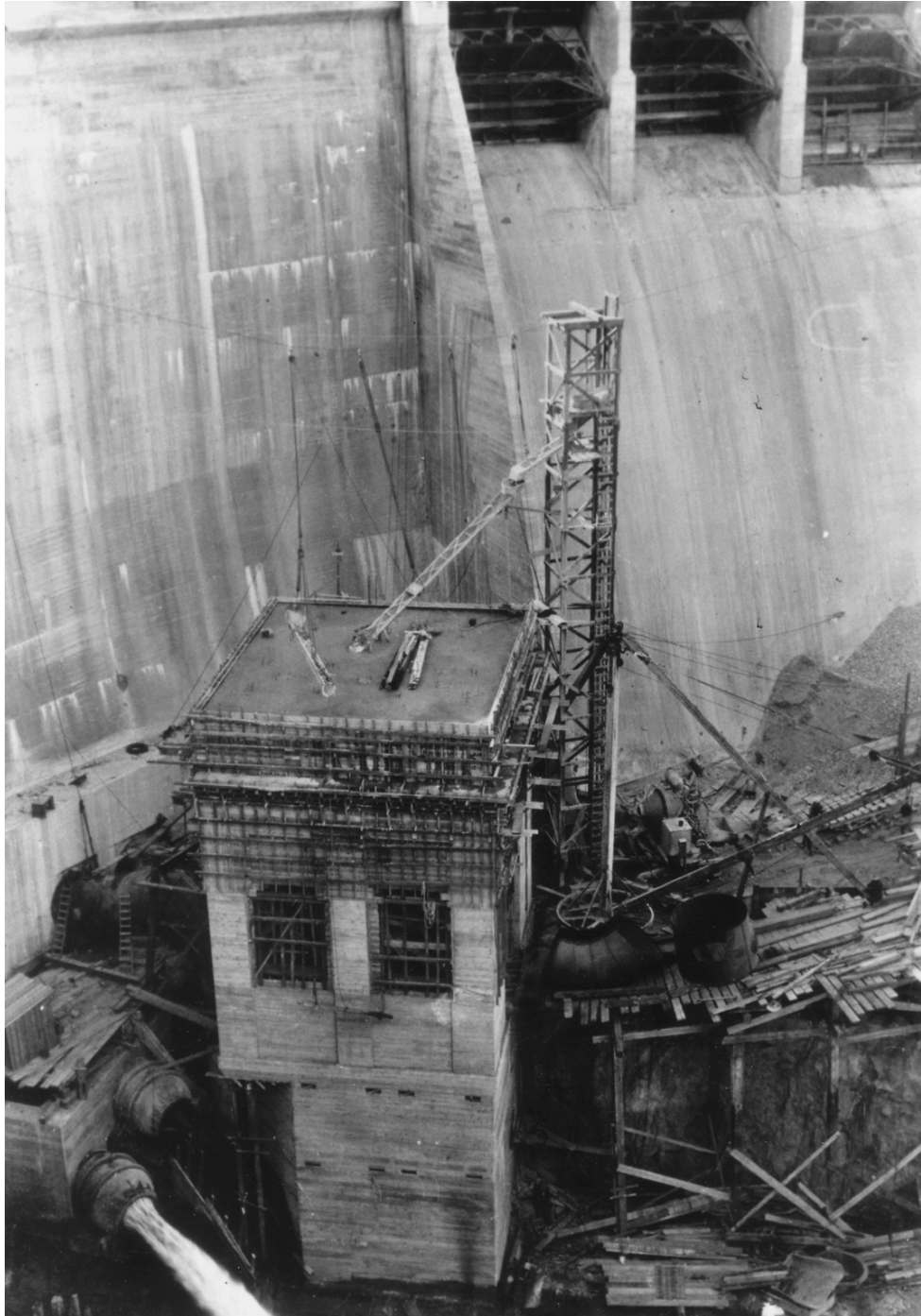
Photo 8: View of the power plant under construction on the downstream side of the dam. Photo taken in March 1926. Note location of spillway gates. Needle valves at lower left are for bypass. Photo courtesy of the SRP.
