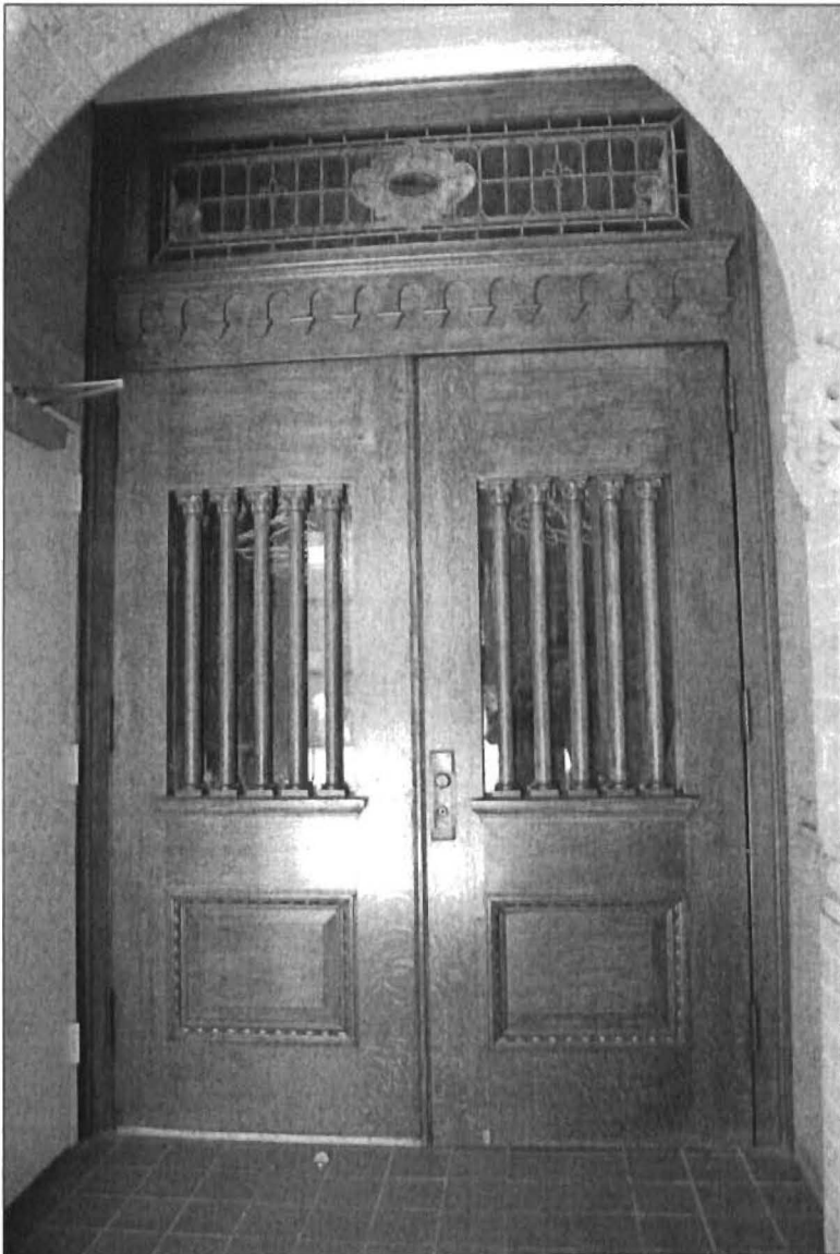
5 of 8. View looking east in the main entrance at original first floor interior entry doors leading to stairway.
