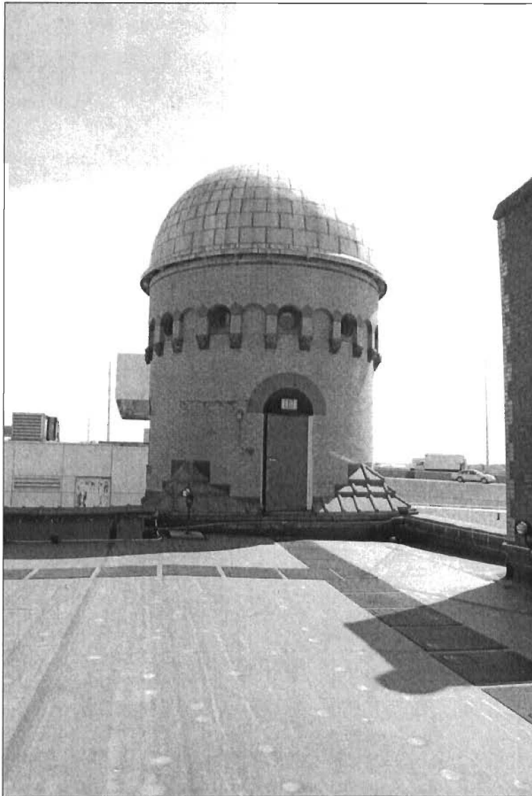
3 of 8. View looking west on the roof at the observatory (elevated highway in background).
