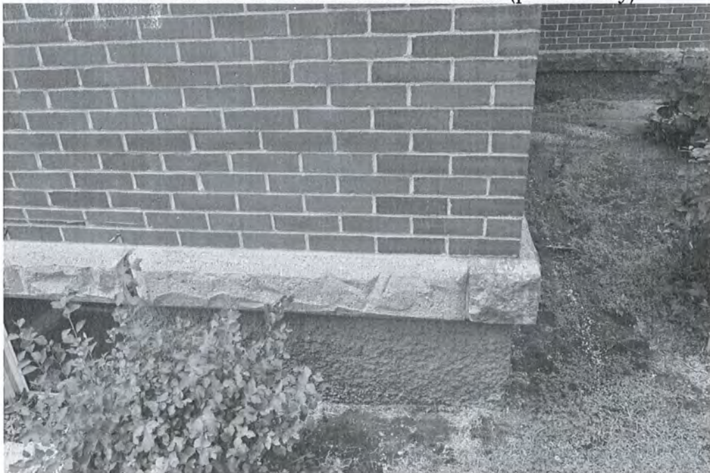
Image 3: Close up of stucco covered foundation and stone foundation cap in General Sherman Hall. In the northeast corner of the addition, one sees the juxtaposition of limestone (at the corner) and textured concrete. (photo Perry)
