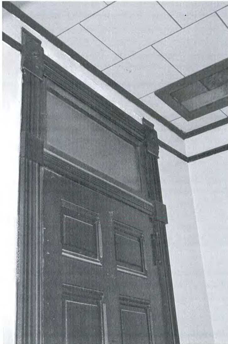
Image 7: General Sherman Hall's original east front wood door and transom are visible inside even though the opening has been covered with brick on the outside. Ceiling opening allows access to the crawl space above. (photo Perry)
