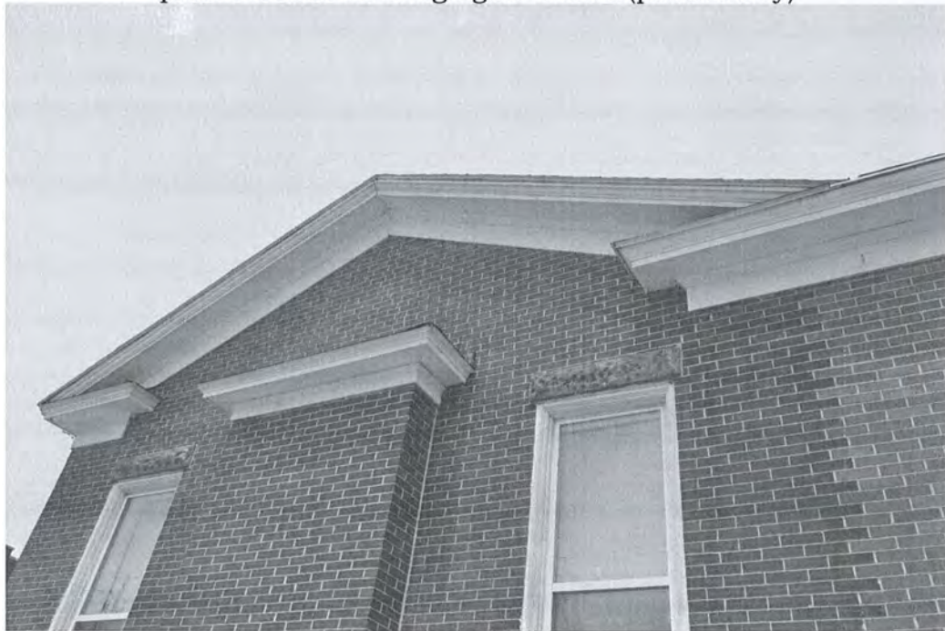
Image 9: Brickwork for 1935 addition to General Sherman Hall is certainly not a perfect match. Limestone lintels are above all windows. (south face of building) (photo Perry)
