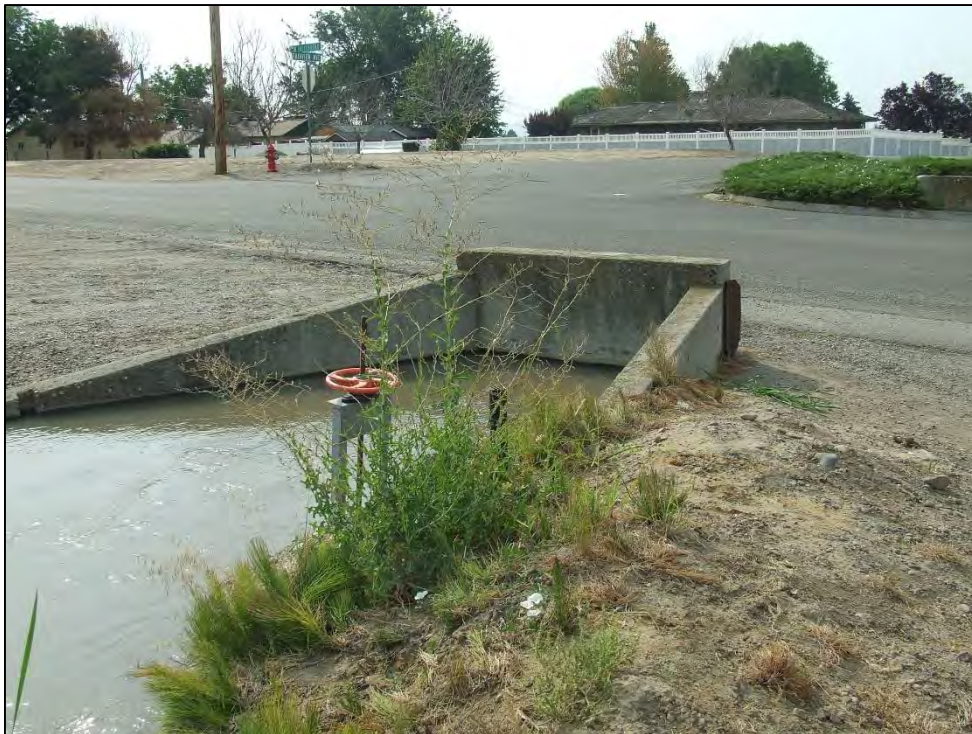
Photograph 24 of 25 Canal at the top of the hill, intersection of Fairview Avenue and Indianhead Road, view looking SE. The water from the pump house comes out in this ditch.
