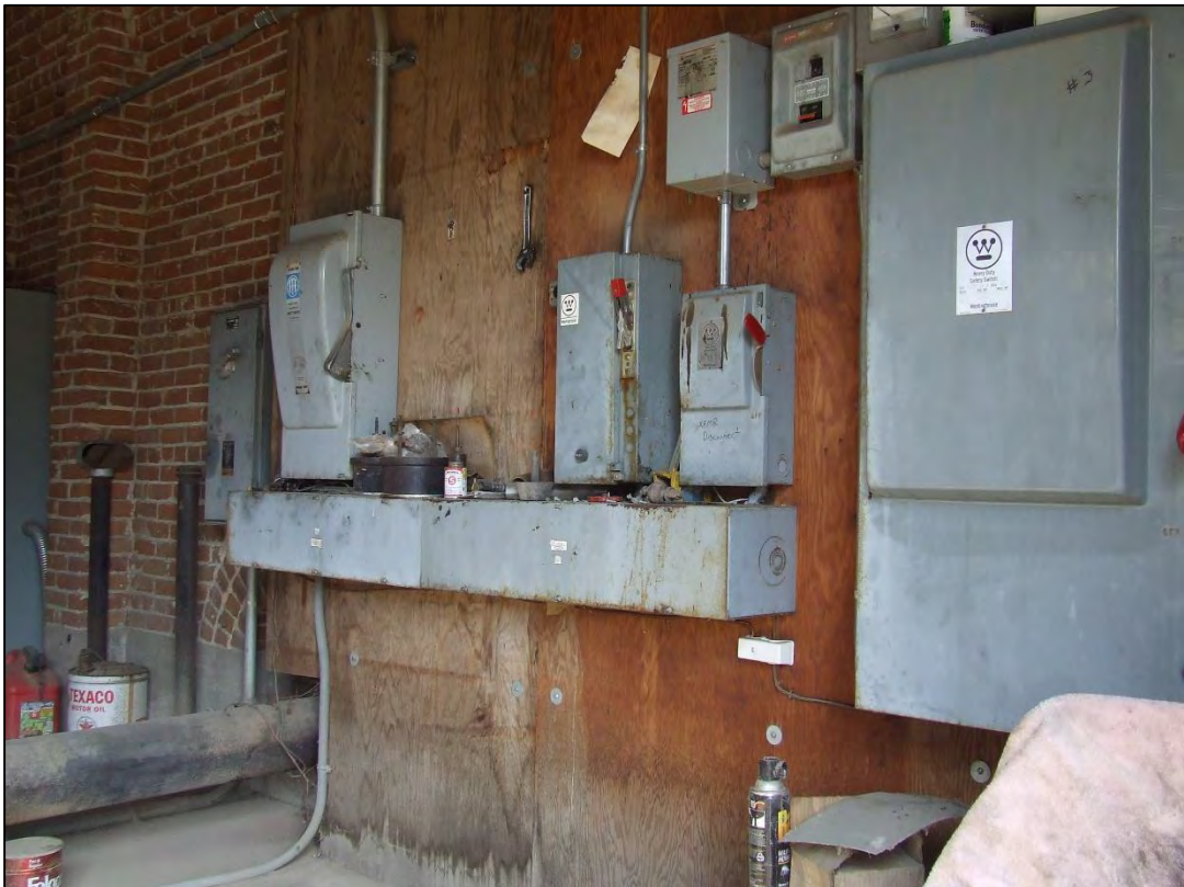
Photograph 22 of 25 Switch boxes mounted on north wall
