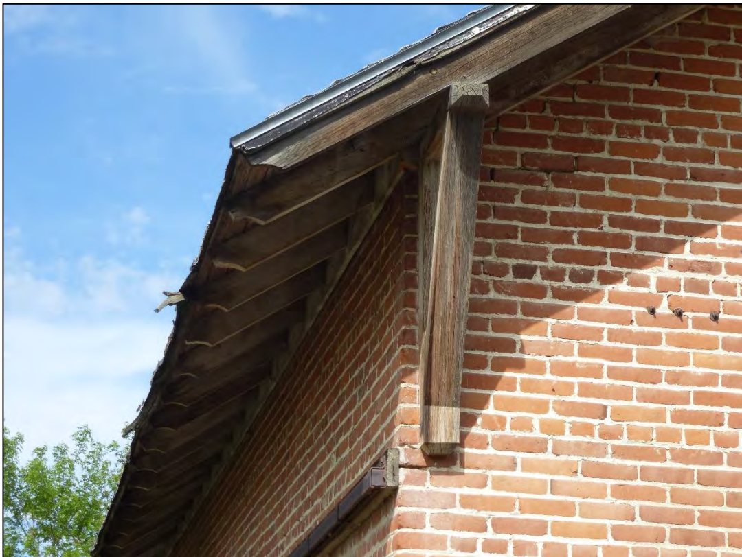
Photograph 8 of 25 Detail view, knee braces and exposed rafter tips, façade and south elevation
