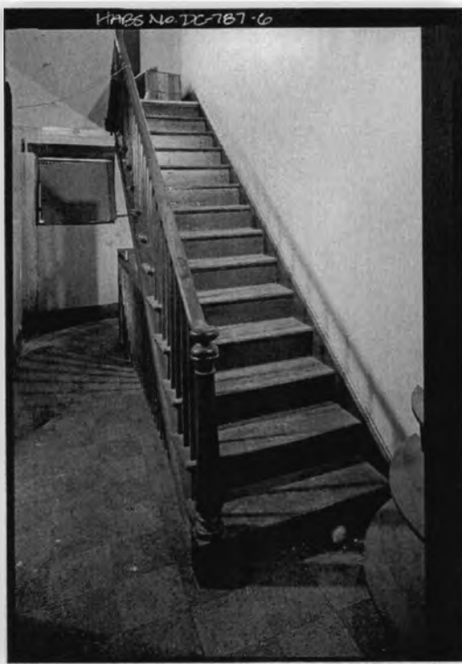
604 H Street NW, Washington, DC, Stairway from Second to Third Floors. 1988. Boucher, Jack. Historic American Building Survey, Library of Congress Prints and Photographs Division. http://hdl.loc.gov/loc.pnp/hhh.dc0913
