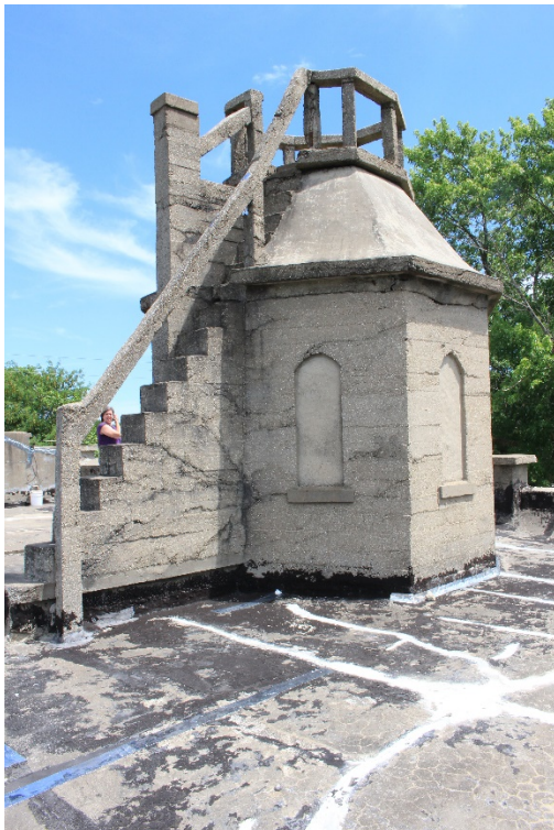
10 of 22: Domed Cupola with Observation Platform and Stairs, Roof. Camera looking southeast.
