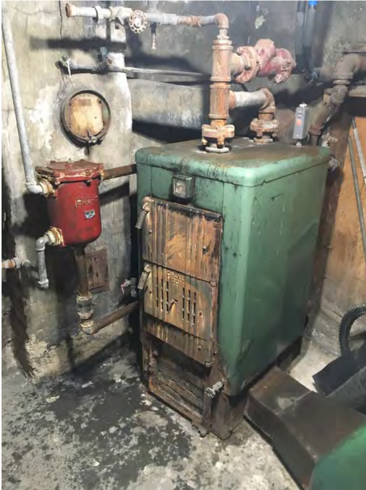
Photo 14. Date: 8/4/2017. Description: Interior, washhouse basement, coal boiler. Camera facing southeast.
