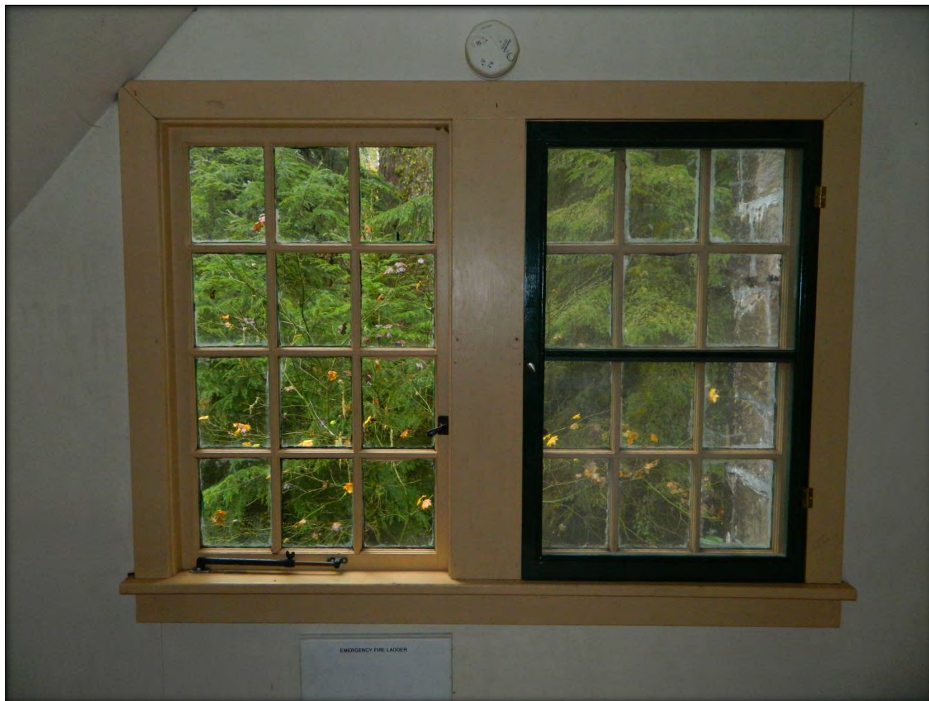
Photograph #24 - Close-up of double twelve-pane wood sash casement windows with mullion. Note the single screen on the right window
