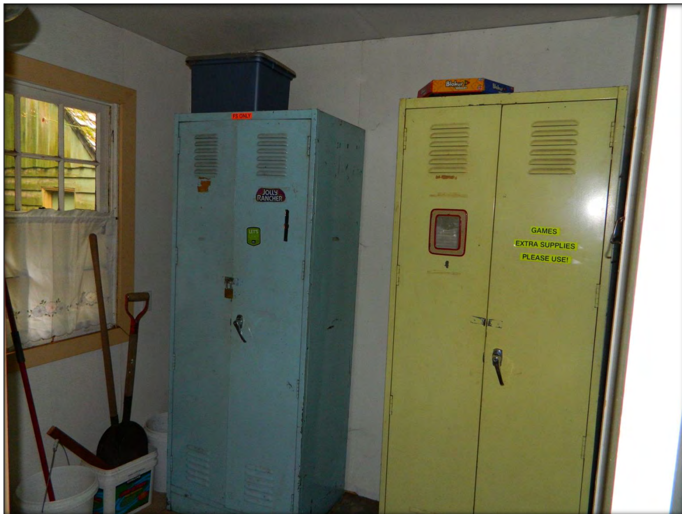
Photograph #19 - Utility Room - former bathroom. With two metal lockers and a single six-over-six wood sash window
