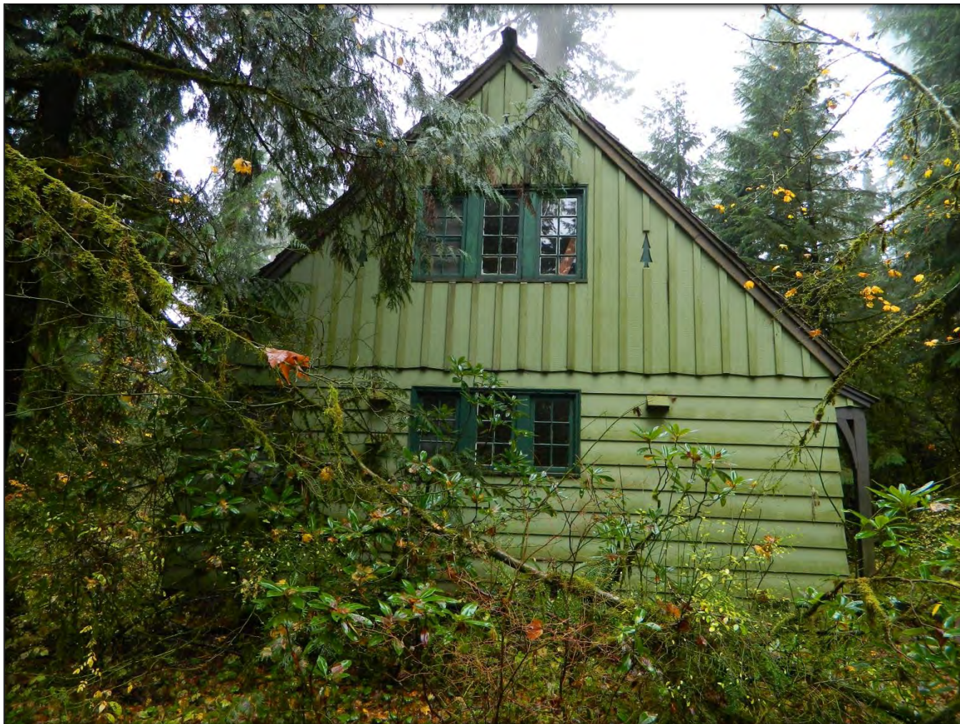
Photograph #6 - Northwest elevation showing gable and windows including window on left not shown on original elevation drawing (Graphics section)
