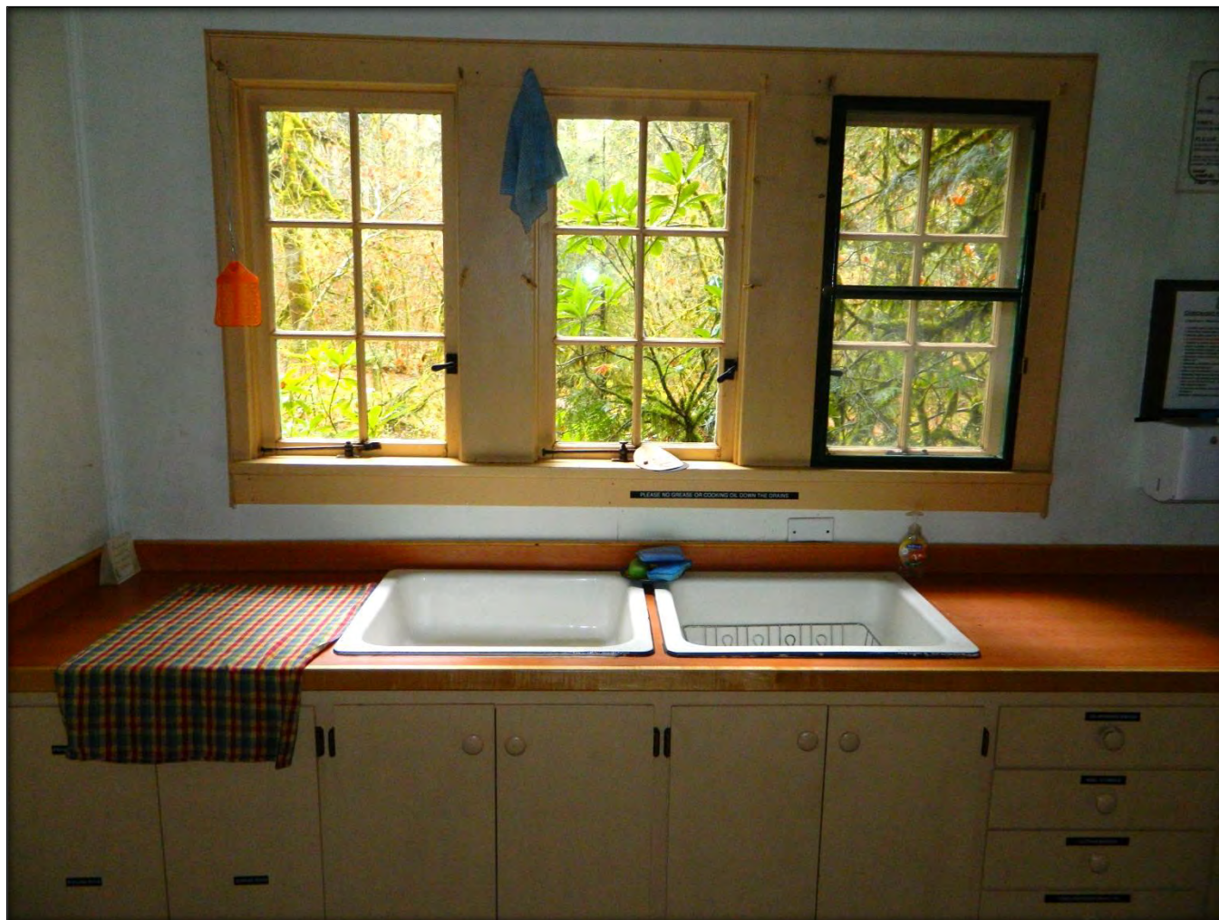
Photograph #18 - Kitchen sink (left) and laundry tub (right) with pine cupboards with plywood doors and spruce counter and back splash. Photo also shows triple six-pane wood casement windows
