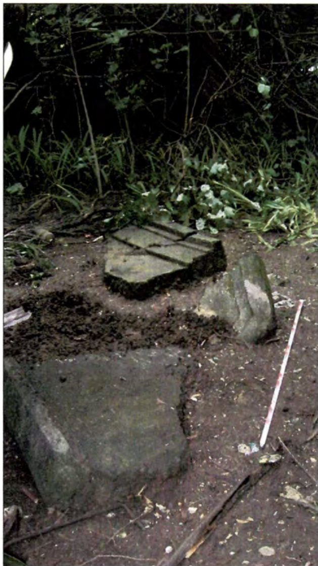
Figure 13. Portions of fallen gable adjacent to the east wall of the building.
