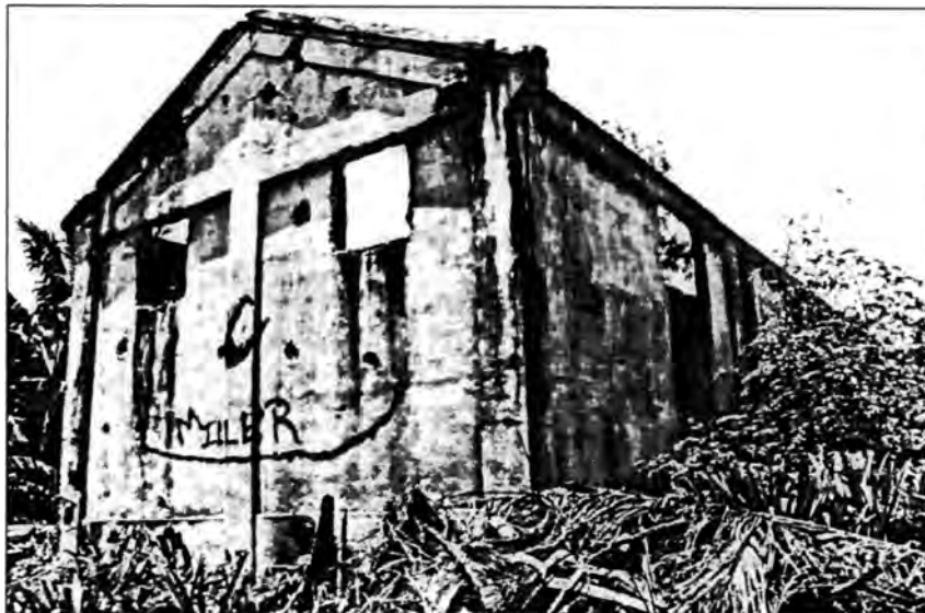
Figure 8. Condition of Japanese Rice Mill in 1983, facing northeast (Kurashina et al. 1983: Figure 15)
