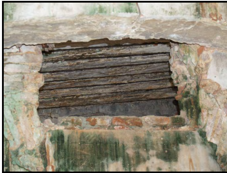
Figure 10. View of the exposed rusted steel rods in the vestry's roof. (Photographer: José Marull)
