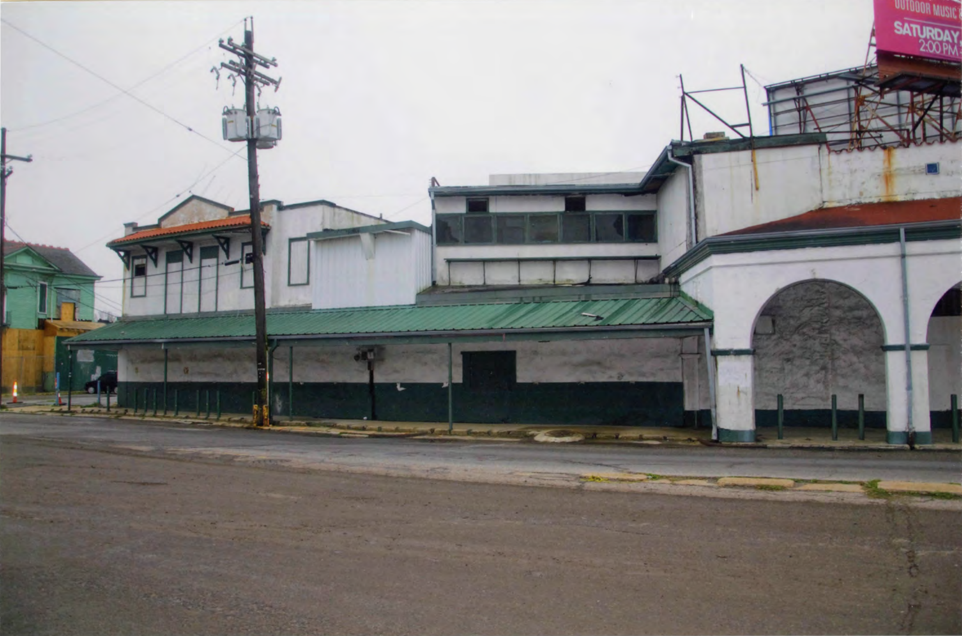
St. Bernard Market New Orleans Orleans Parish Louisiana Photographer John Williams February 2012 St. Bernard Elevation - Camera Facing SW Photo 0001
