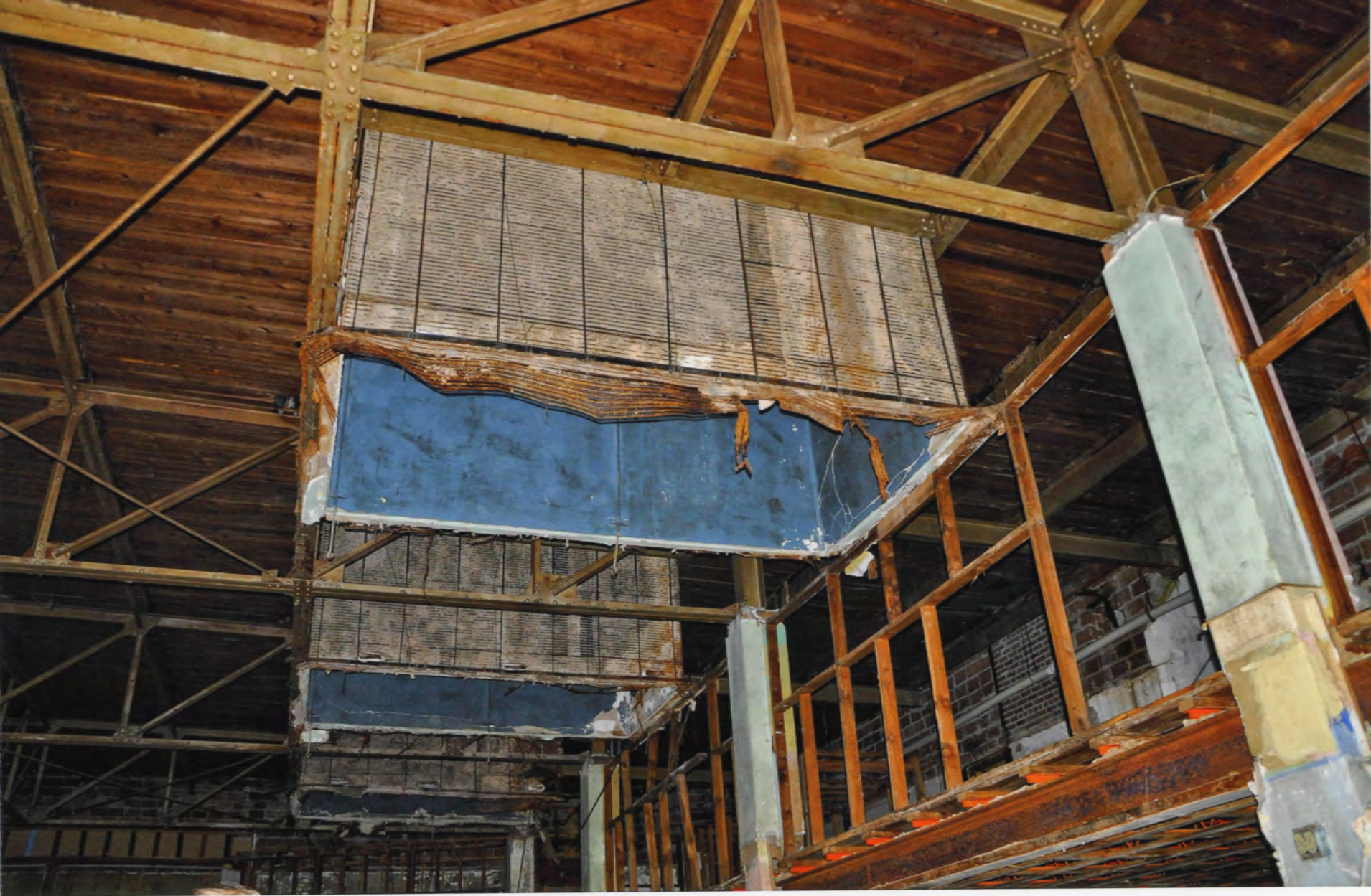
St. Bernard Market New Orleans Orleans Parish Louisiana Photographer John Williams February 2012 Light Monitor Detail - Camera Facing SW Photo 00021
