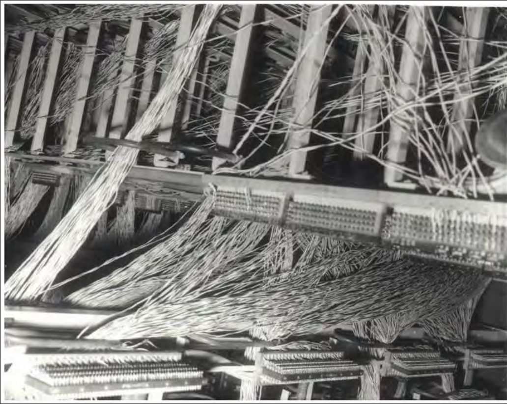
Figure 5. Wires for telephones in the United Telephone Building. From the High Plains Museum ( https://i2.wp.com/highplainsmuseum.org/wp-content/uploads/2012/04/presentation3.jpg )
