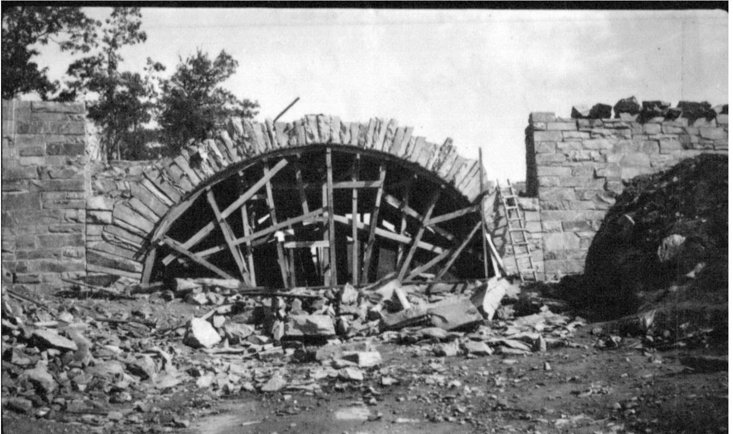
Figure 16. Construction of the May View Drive overpass structure at U.S. 221, September 1938. Photographer unknown; photograph courtesy of National Park Service, Blue Ridge Parkway.
