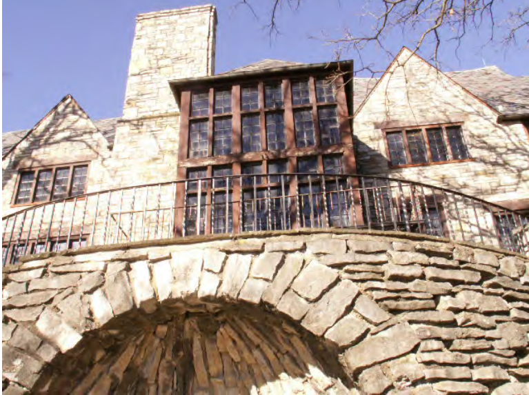
Fig. 7 of 43: Rear chimney, camera facing northwest, Photograph Taken by Nikole Meyer ca. 2016
