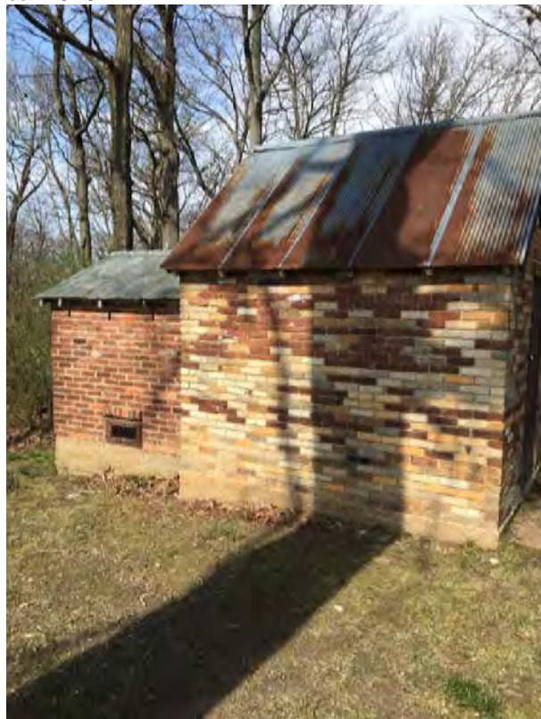
Fig 30 of 43: Southern elevation of smokehouse, camera facing north, Photograph Taken by Nikole Meyer ca. 2016
