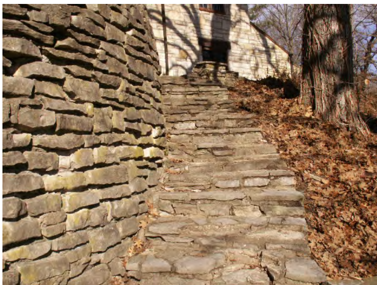
Fig. 13 of 43: Outside staircase, camera facing west, Photograph Taken by Nikole Meyer ca. 2016
