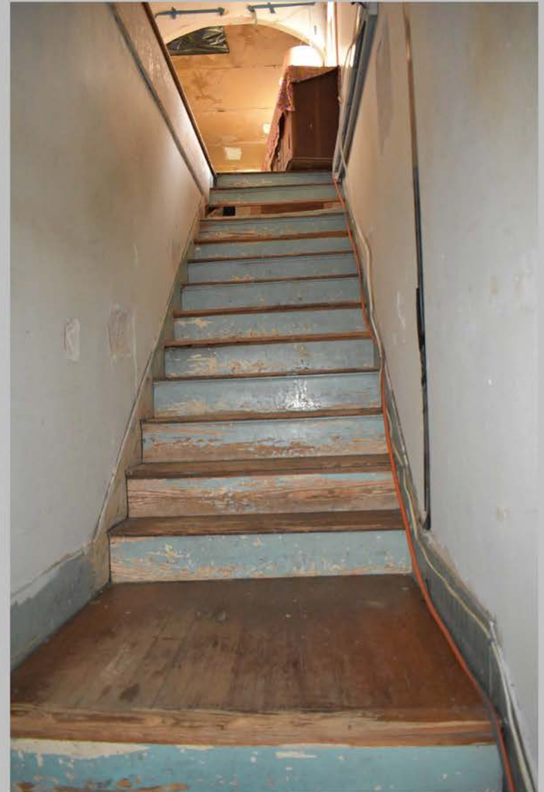
4. Stairs from first story entry to second story living space, looking southwest.
